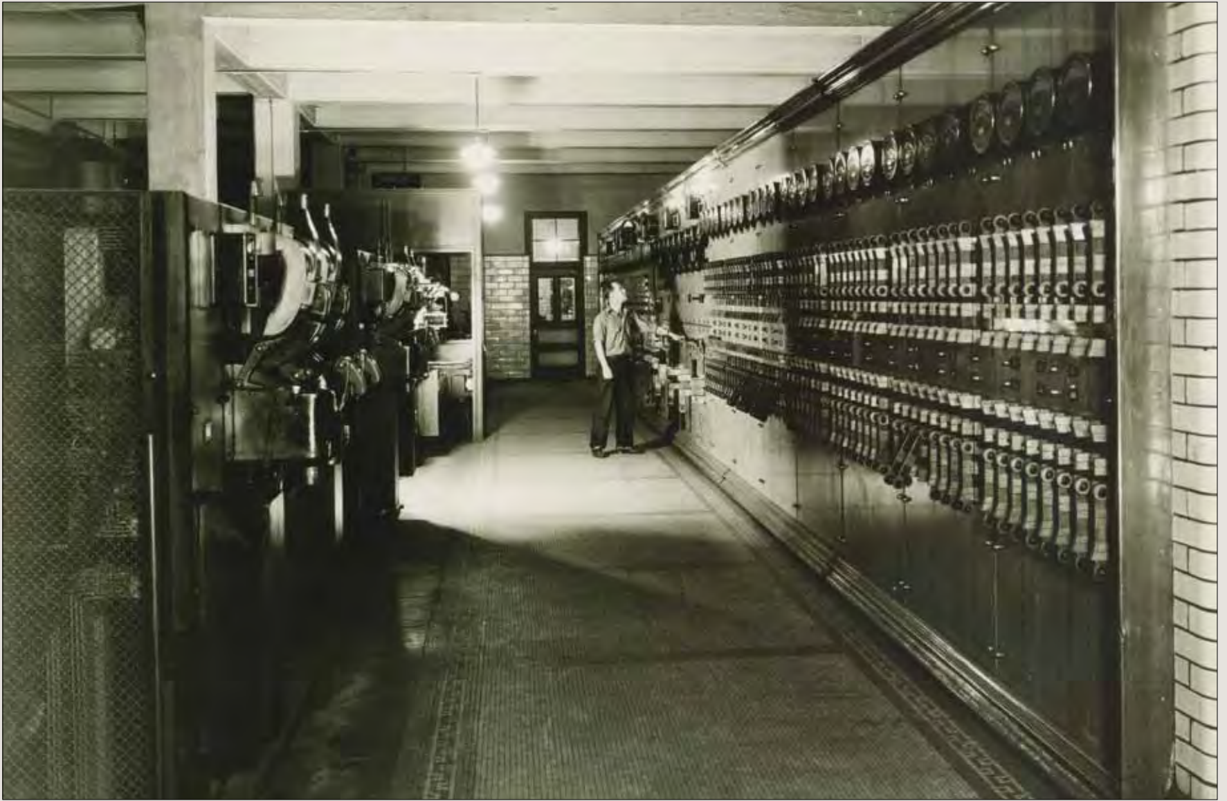
These switchboards controlled the distribution of electrical power to circuits throughout the buildings. Photo circa 1930.
