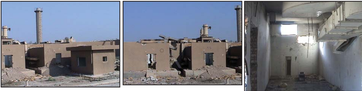
Figure 15. Damage at Ash Shaykhili Building 27B and remaining air ducting in July 2003.
