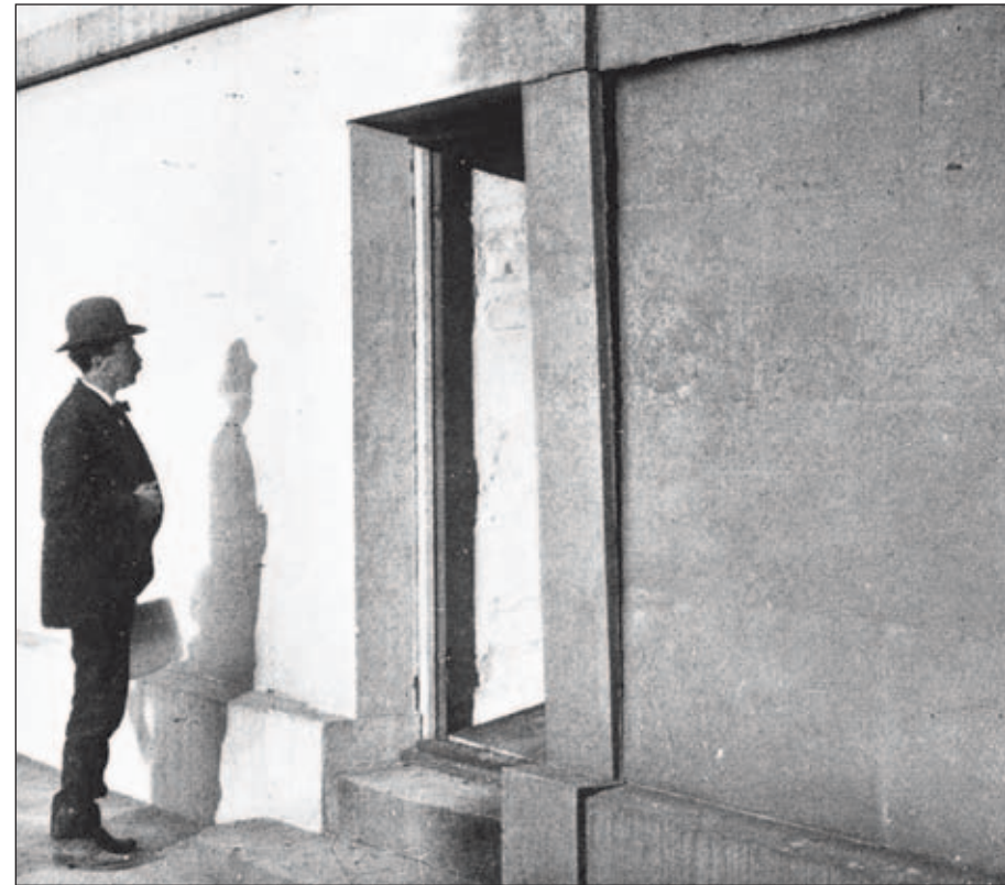
Figure 12. Brown inspecting damage to the Capitol's west wall after the 1898 gas explosion.
