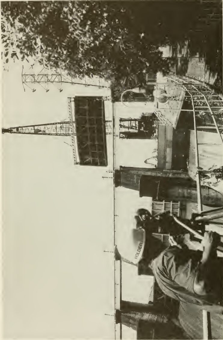
The floating crane GOLIATH removes a flood gate during the first major overhaul of Miraflores Spillway. A Commission photographer captures the event on film to document the procedure and prepare instructional films to aid in future maintenance training programs.
