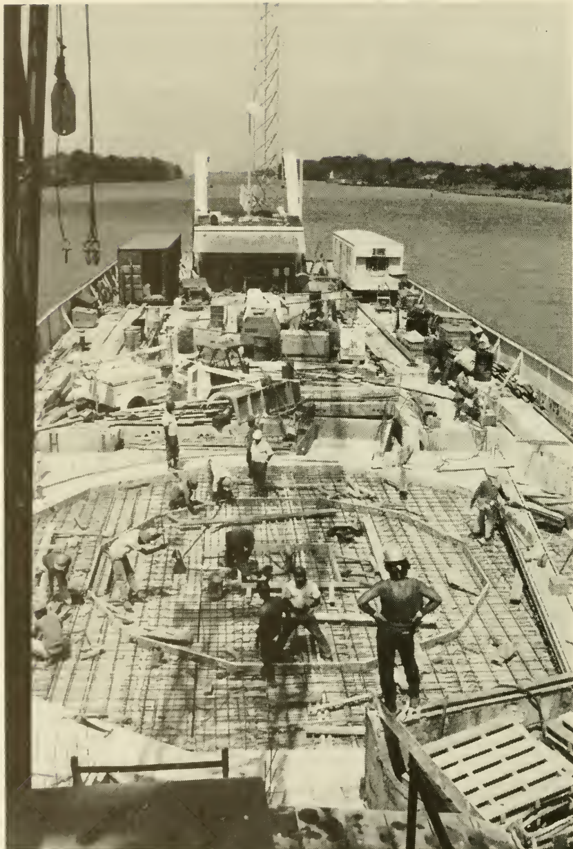
Workmen prepare the foundation for a new towing locomotive turntable at the north end of the Gatun Locks center wall. This is part of an ongoing project to replace towing locomotive turntables at all locks to allow earlier attachment of locomotive wires to transiting vessels for improved control during lockages.
