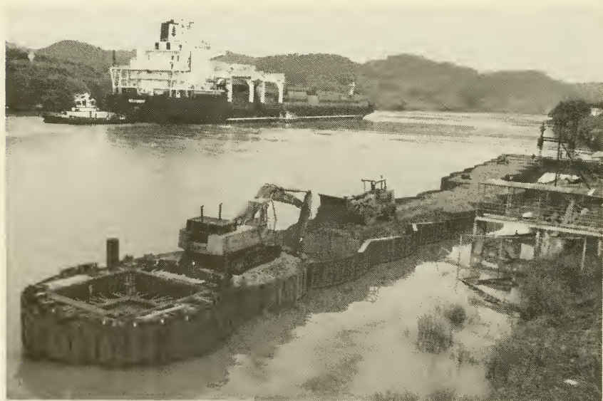
A contract was awarded to upgrade the former floating wooden landing at the Paraiso tug and launch facility. Construction work can be seen in progress (upper photo) as the Panamax-size vessel BELFOREST transits in the background, heavily laden with lumber products. The new permanent concrete facility (lower photo), which was completed on August 25, 1992, requires little maintenance.
