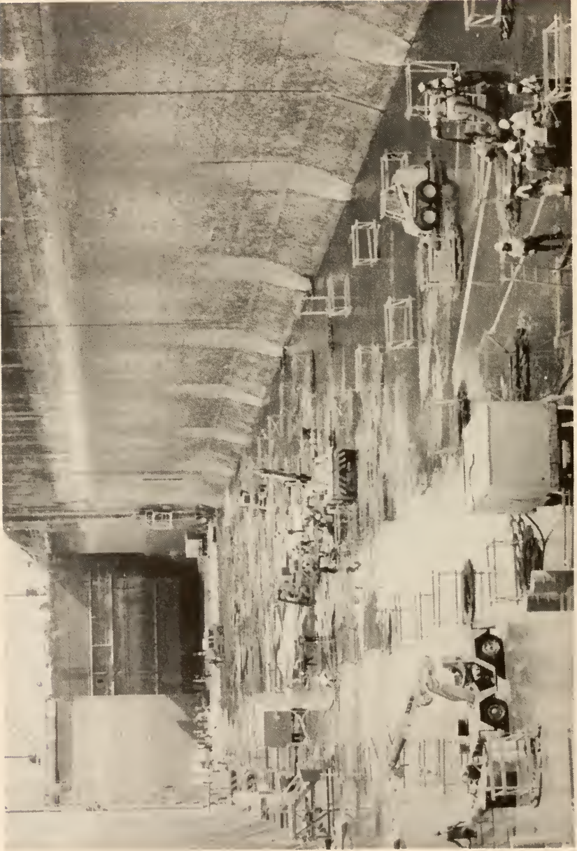
Craftsman labor on the floor of Pedro Miguel Locks performing essential structural inspection and repair of all culverts, valves and miter gates during overhaul. Planned maintenance continues to be the key to the operational effectiveness of the Panama Canal.
