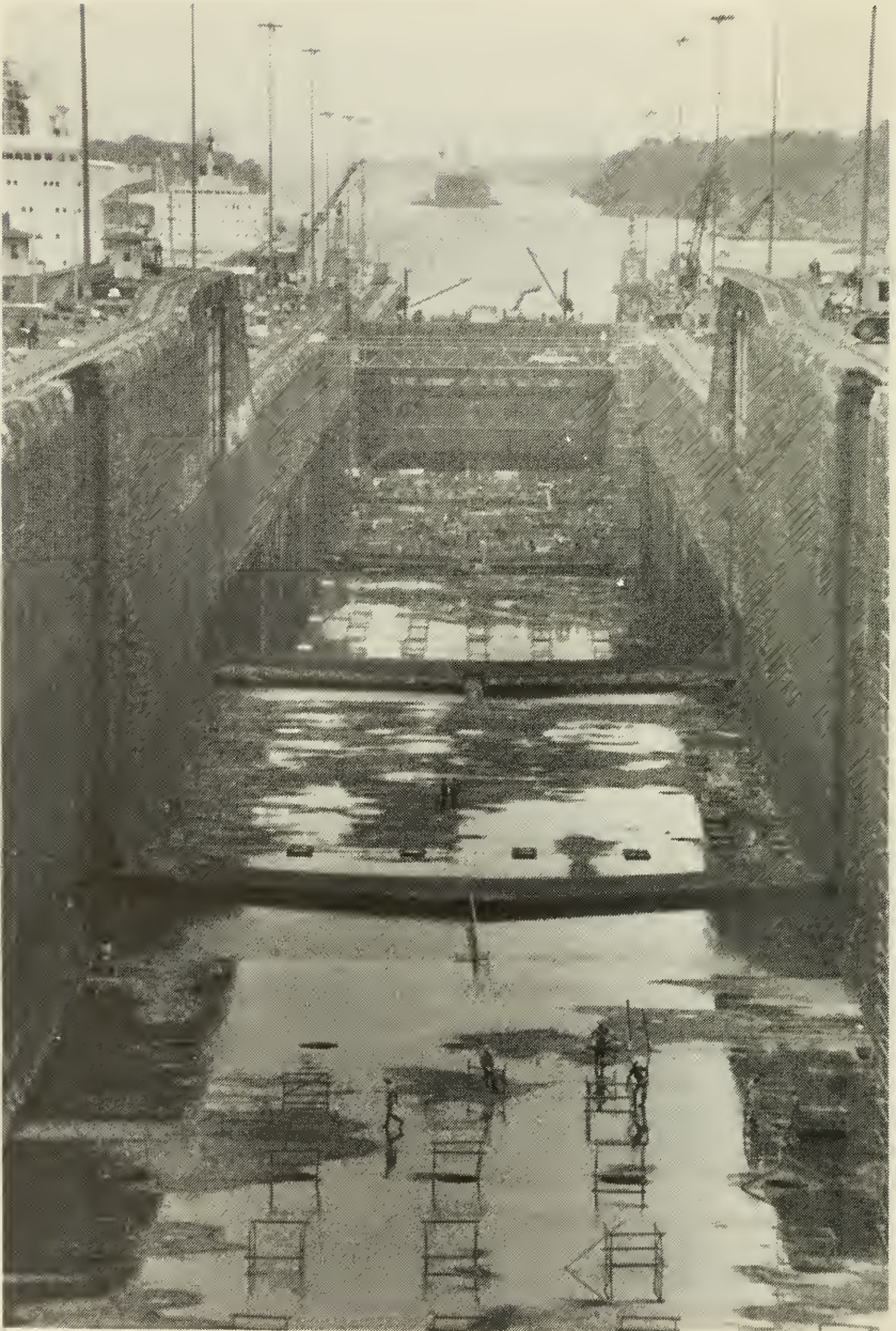
Dry chamber work is performed at Gatun Locks while vessels continue to transit the Canal utilizing the alternate lane. Two vessels can partially be seen to the left during lockage operations while another vessel approaches Gatun Locks. More than 13,000 vessels pass through the Canal each year.
