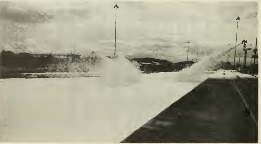
Tests were conducted on the new foam fire fighting system installed at Miraflores Locks. The system consists of eight remote controlled foam nozzles located strategically at the forebay and tailbay areas of the locks. Upper photograph shows the northeast lane filled with foam following the test. Lower photograph shows the test in progress.
