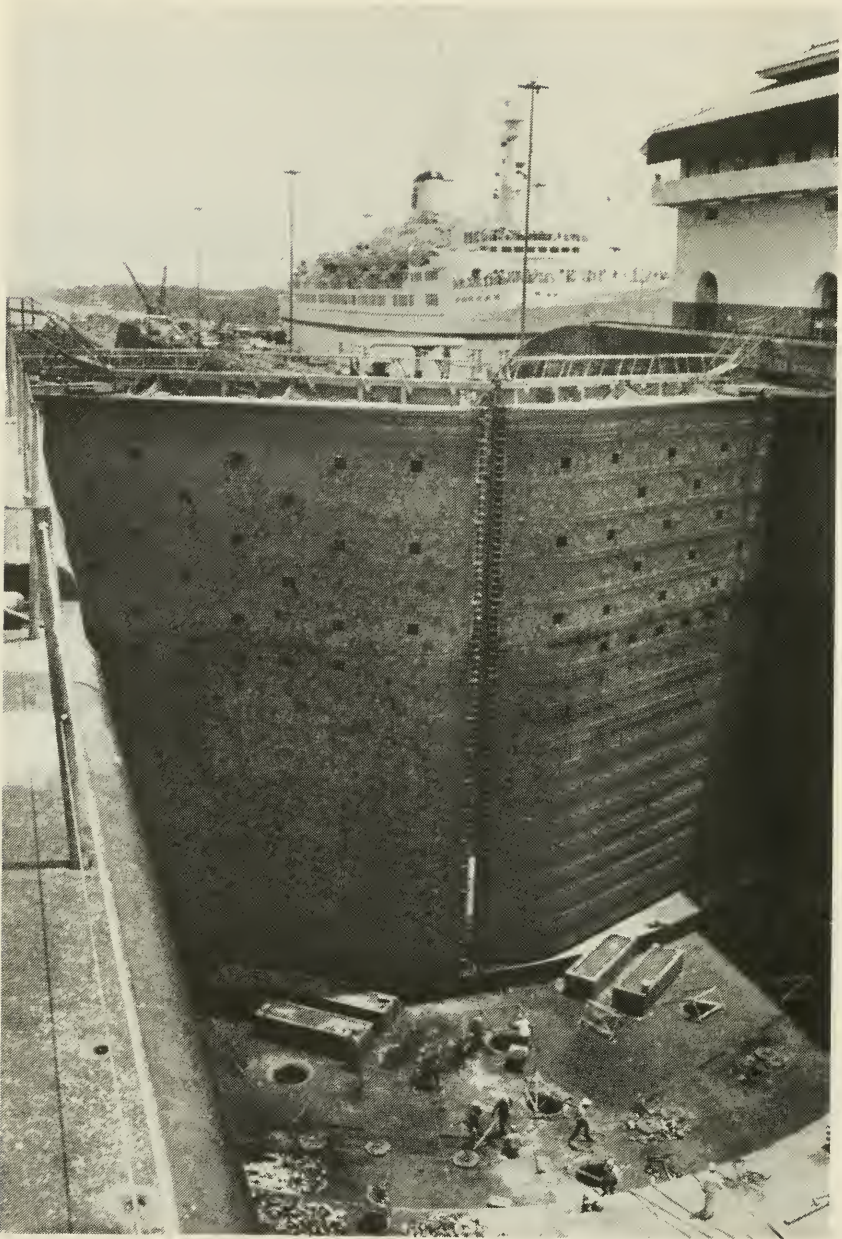
From the comfort of a luxurious cruise ship passengers view dry chamber work in the west lane of Gatun Locks during an overhaul. This $7.4 million project included removal, rehabilitation and reinstallation of four miter gates; maintenance work on rising stem valves and the locomotive tow track system; and repair or replacement of fendering and cathodic protection.
