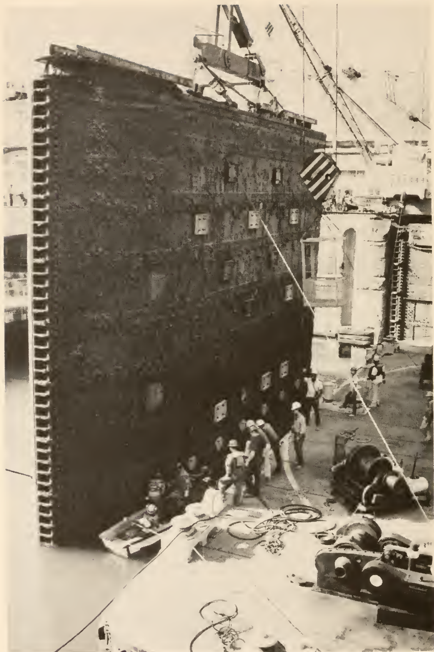
One of four massive 750 ton sea gates, removed during the Miraflores Locks overhaul, is partially lifted from the water by the floating crane HERCULES to allow workmen to seal closure plates. The gate was then floated and towed in barge-like fashion to the Mt. Hope Industrial facility for thorough overhaul. Major maintenance efforts such as this are critical to the effective and efficient operation of the Canal's lockage system.
