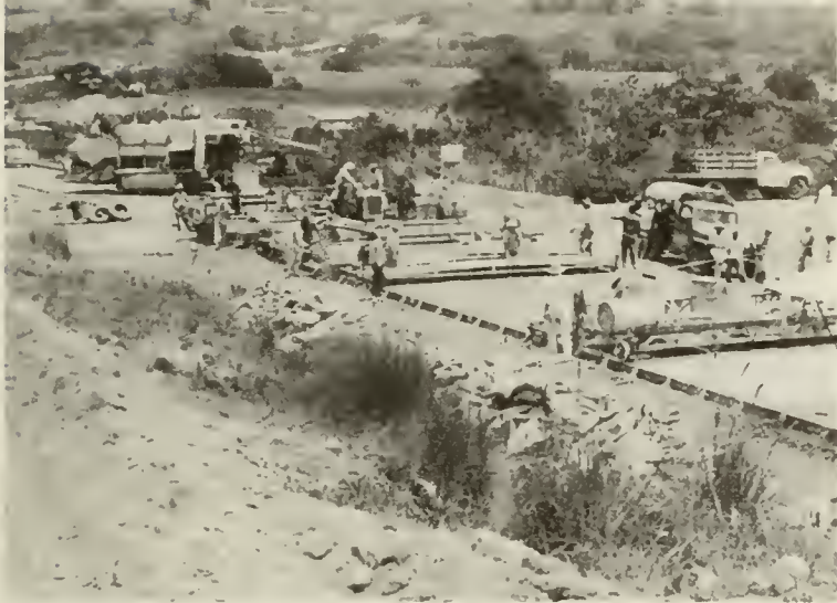
Paving machinery and crews at work on Inter-American Highway sector near Tolé, looking east, the direction in which paving work is progressing.
