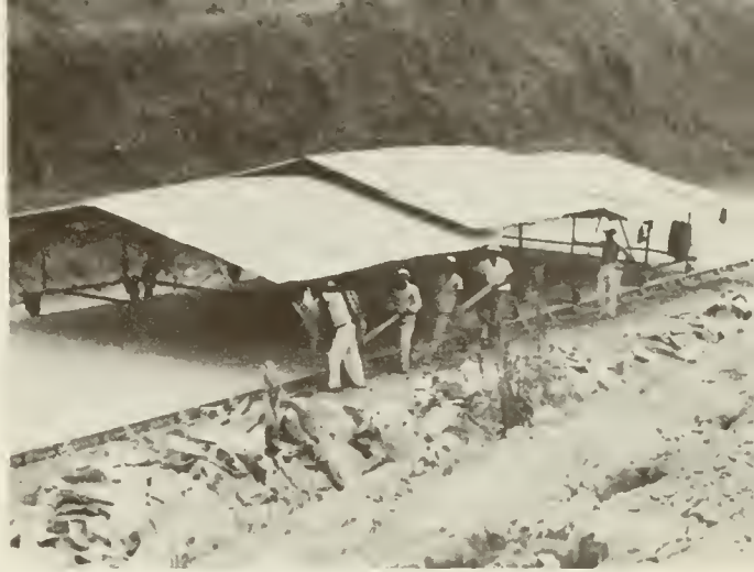
Rolling "roof" for freshly poured concrete. It keeps rain or sun off to protect the material during first stage of setting. One of these is with each paving machine.
