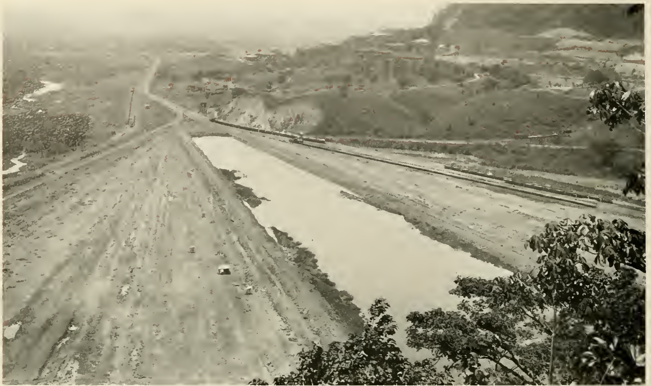
Clearing and leveling land for construction of the townsite of Balboa and the Canal Administration Building was underway when this picture was taken from atop Sosa Hill in June, 1912.
