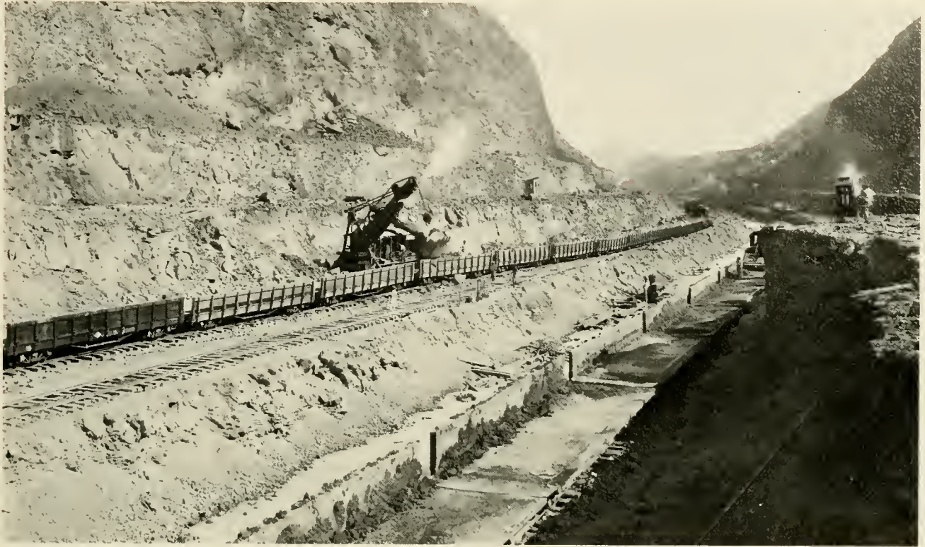
Dirt trains are loaded in Culebra between Gold Hill and Contractors Hill, December 28, 1912. To the left of the flat cars is the bottom of the Canal.
