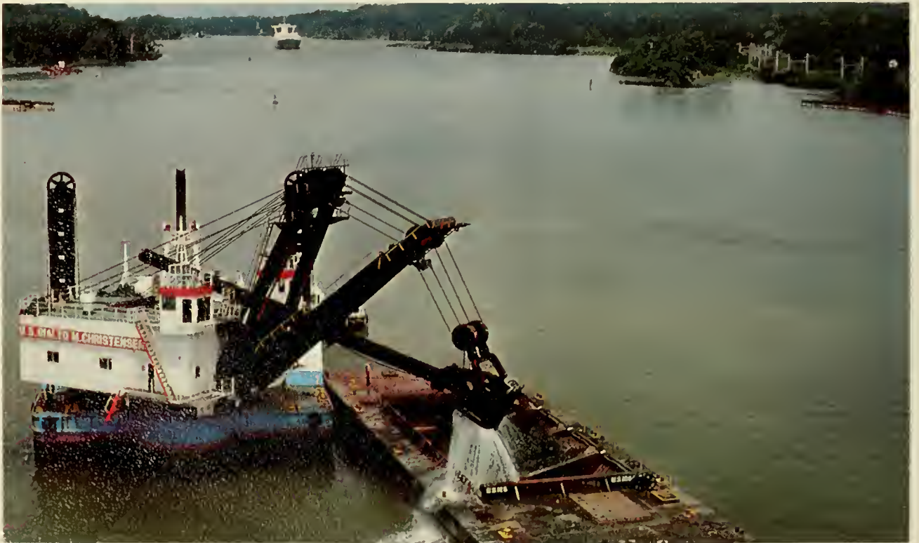
Dredging is still an integral part of Canal maintenance. The Panama Canal Company recently added to its fleet the $6 million "U.S. Rialto M. Christensen", the largest dipper dredge in the world.
