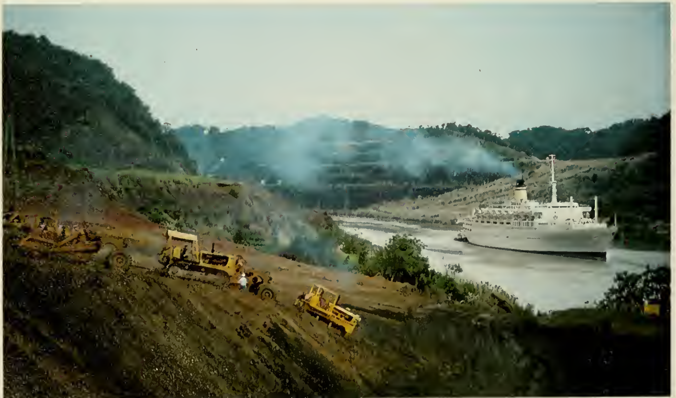
Work on clearing of the slide that occurred October 10, 1974, continues as a cruise ship passes through the Cut.
