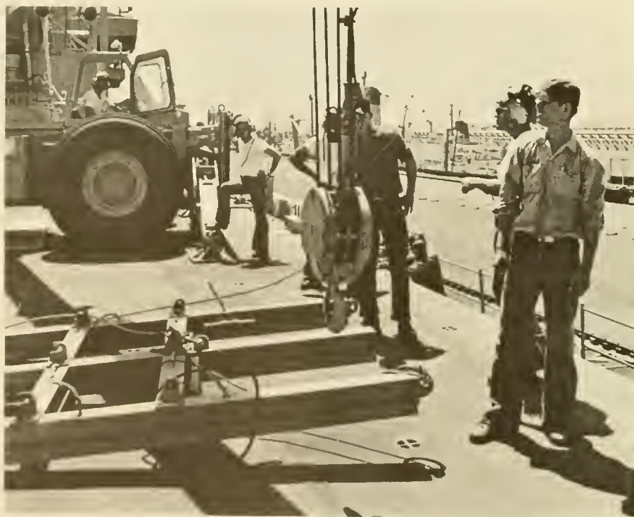
Protrusions are removed from the vessel to make it possible for her to transit the Canal. The work was performed in Cristobal by the Industrial Division.
