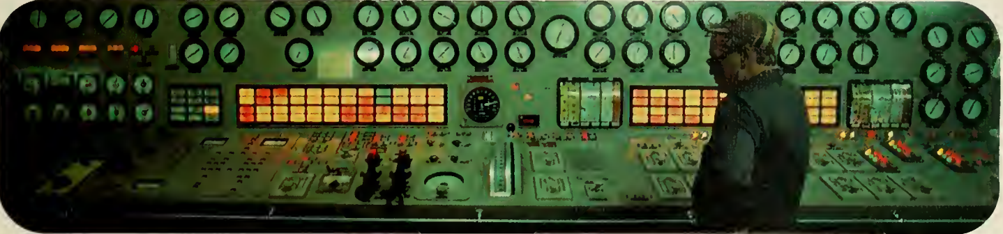
Activity in all cargo holds can be observed quickly on this highly automated control board.
