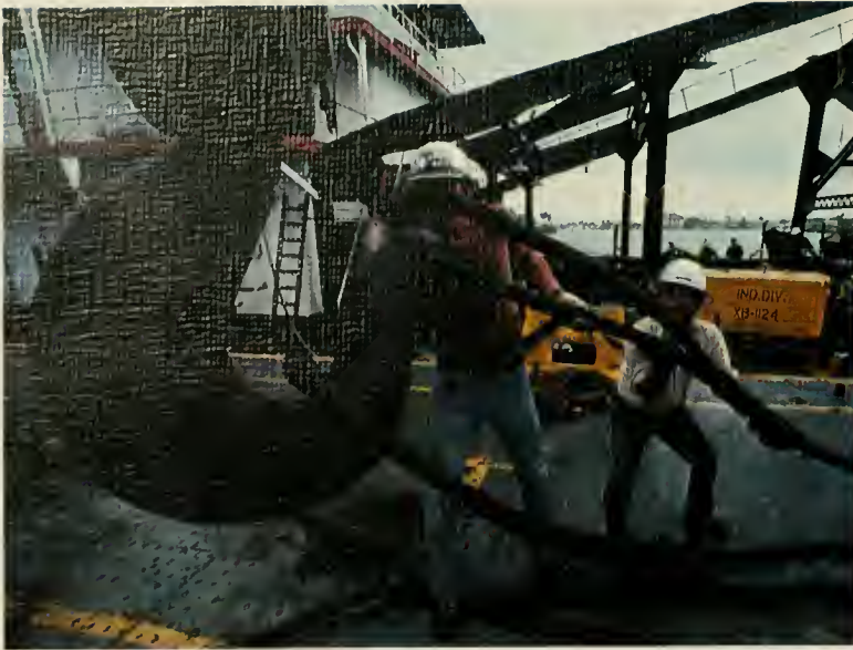
Workmen are dwarfed by the huge hook of the "Hercules" as they loop one of four cables that will enable the crane to raise the 160-ton structural steel ladder from the dredge "Mindi" at the Industrial Division in Mount Hope. The "Hercules" and its sister the "Ajax" were built in Duisburg, Germany at the start of World War I. Tradition has it that at the request of the U.S. Department of War, hostilities were delayed for 3 days to allow the floating cranes to pass through the British blockade and proceed to the Panama Canal.
