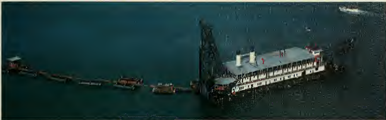
The suction dredge "Mindí" sucks up the continuous accumulation of silt in Balboa harbor capable of restricting the draft of vessels and pumps it outside of the channel.
