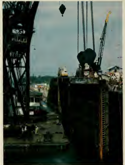
The 250-ton capacity crane "Hercules" is the Canal's only piece of floating equipment capable of lifting the 700-ton locks miter gate off its pintles for overhaul. The buoyant gate is raised into a horizontal position in the full locks chamber and floated to a drydock for maintenance.
