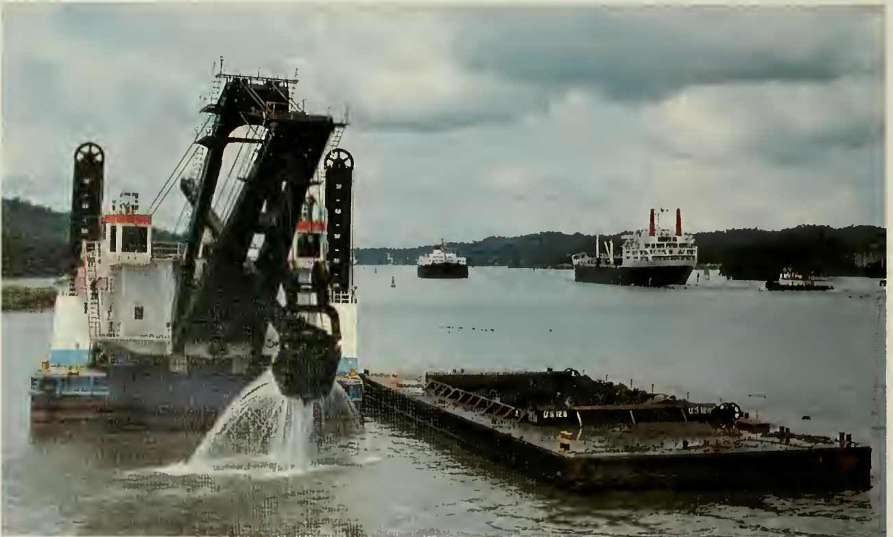
One of the largest dipper dredges in the world, the "Rialto M. Christensen" dredges alongside Santa Cruz Island at Gamboa as part of a Canal widening project. The dredge's 15-cubic yard bucket empties into a scow which will be pushed by tug to a dump site.
