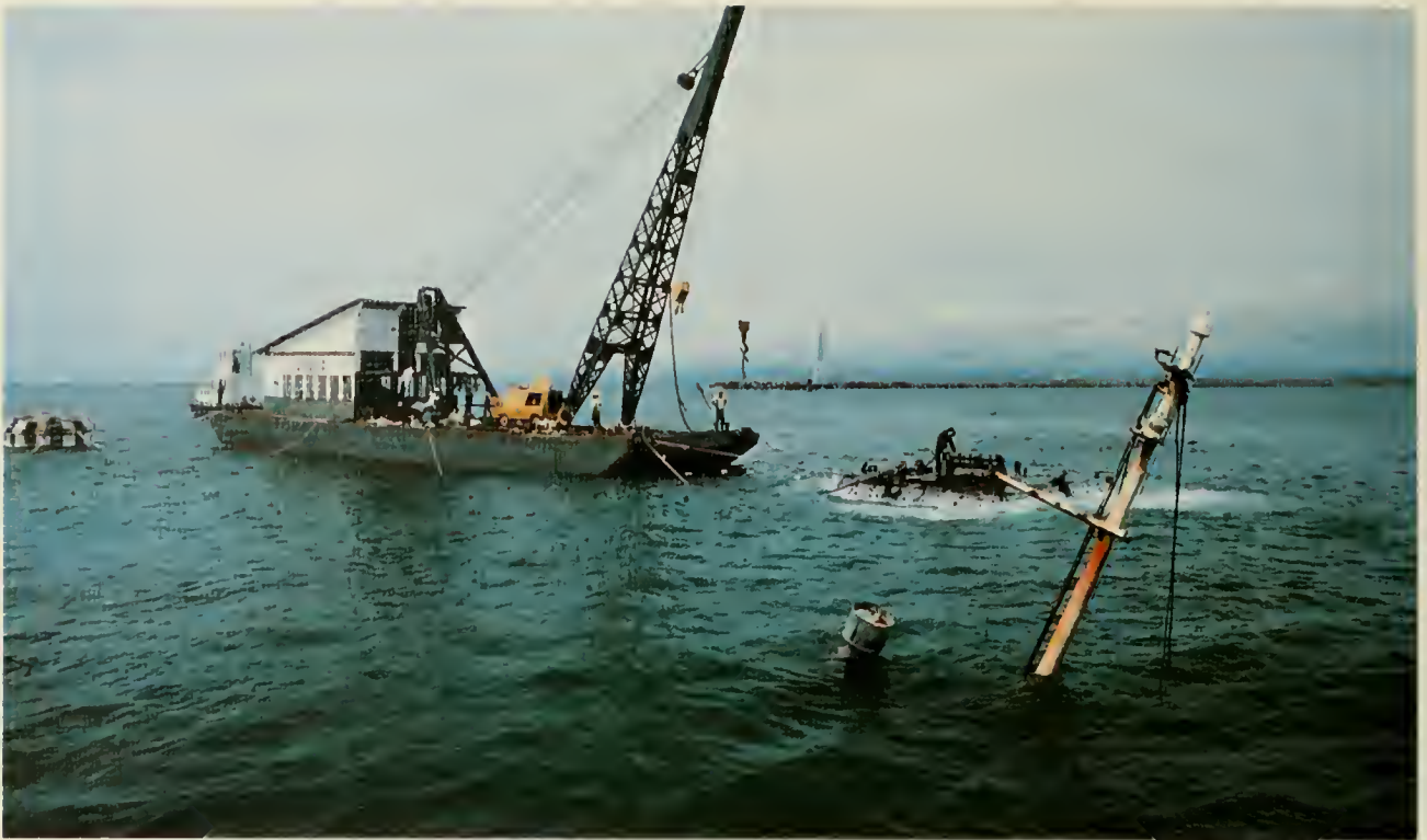
An anchor barge positions one of the huge steel pontoons used in an attempt to raise the Colombian cargo ship "Tairona" after it sank in 44 feet of water at the entrance to Cristobal harbor.
