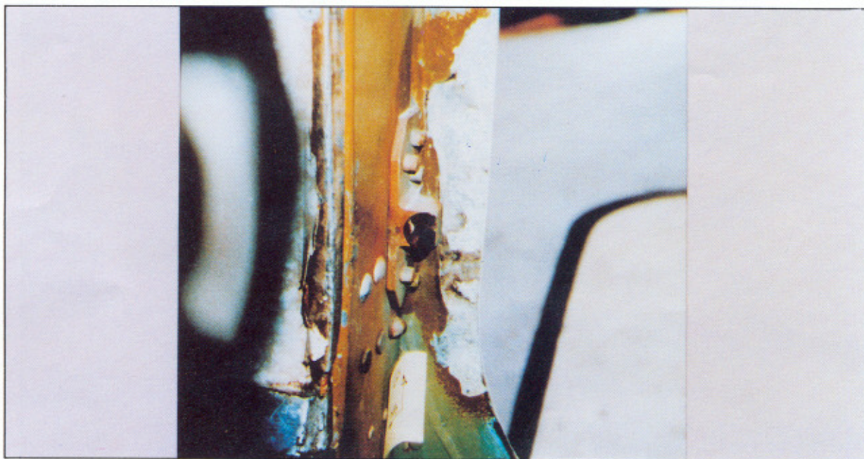
FIGURE 5-12. CORROSION DEVELOPED UNDER LEVELING COMPOUND INSTALLED DURING PREVIOUS REPAIR OF OVERWING EXIT
