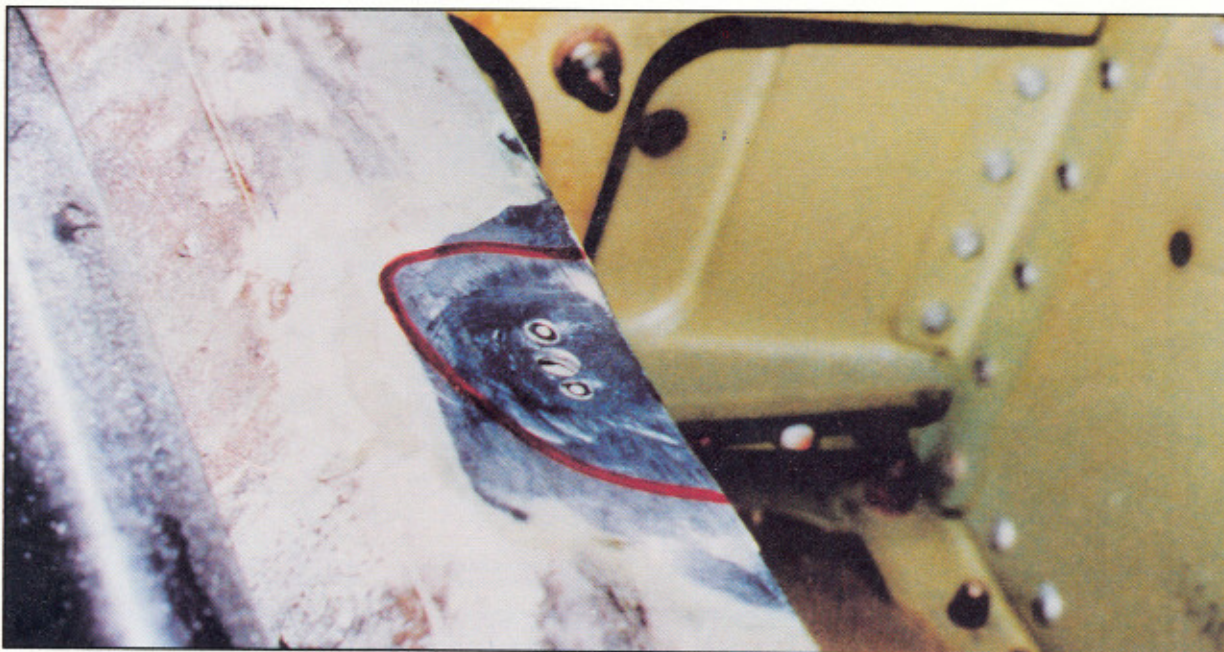
FIGURE 6-5. STEEL PARTICLES FROM FASTENERS OR NUTPLATES MAY CAUSE FUTURE CORROSION PROBLEMS IN ALUMINUM STRUCTURE
