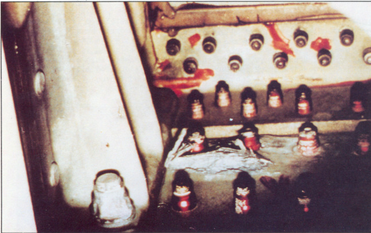
FIGURE 2-9. SEVERE EXFOLIATION CORROSION
