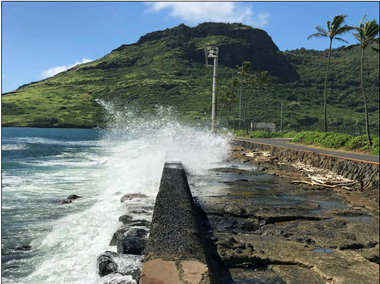
Figure 7.23. Wave overtopping a seawall (Lihue, Hawaii, 2018)
