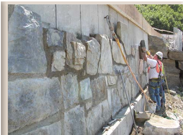
Masonry workers are attaching a historically compatible stone veneer to a new concrete retaining wall near Triple Aches.
