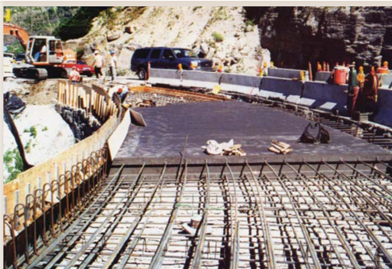
As shown in this photo, more durable and longer-lasting reinforced concrete pavement is being installed in rockslide and avalanche-prone areas such as this site just east of Triple Arches.
