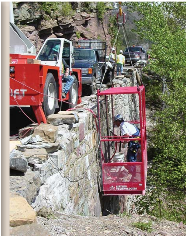
Many retaining walls, like this one near Crystal Point, are being "repointed," the process of removing and replacing damaged and deteriorated mortar. Here a crane lowers a worker, enclosed for safety in a cage-like basket, to perform repairs.
