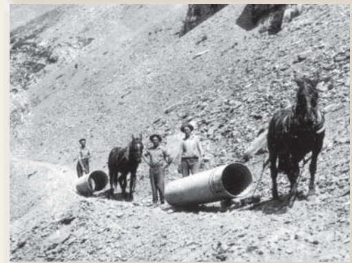
Workers drag drainage pipes by horseback in 1927 during construction of the road west of Logan Pass.
