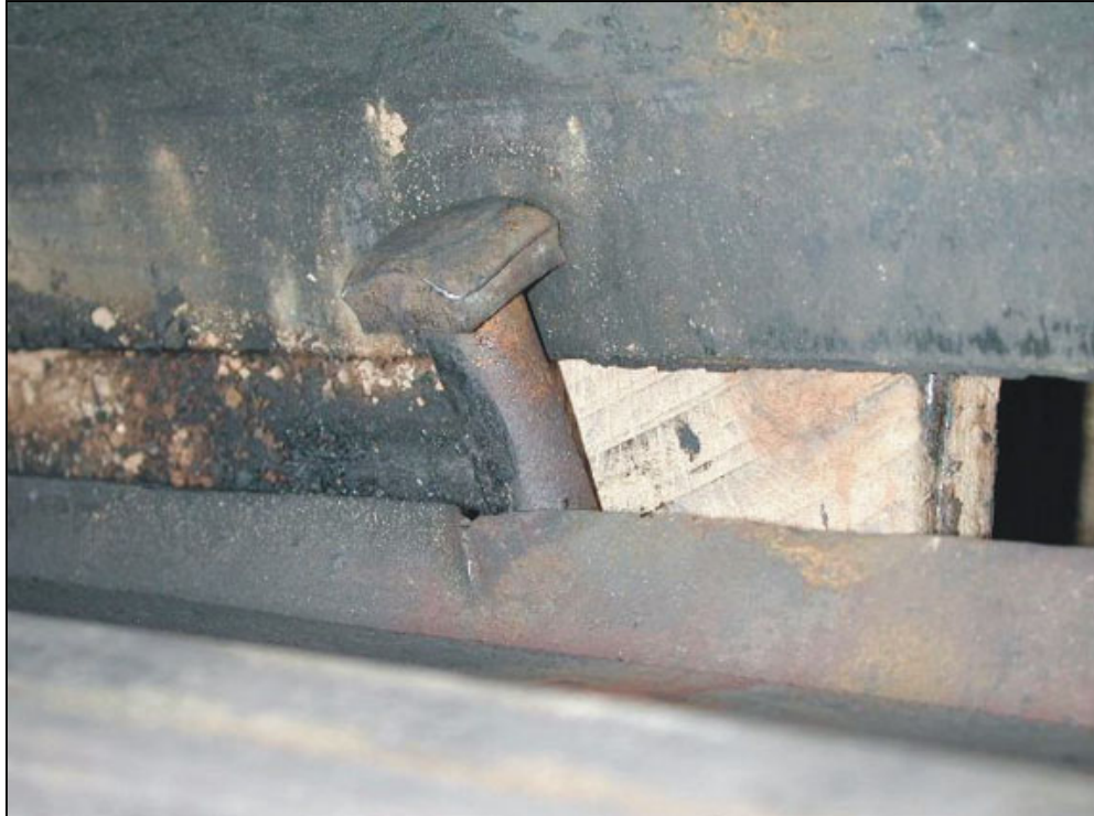
Figure 5. Postaccident reconstruction of broken bolt section as positioned before the derailment.
