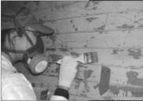
Workman cleaning a barrack wall. Using SAT funds, paint and putty were removed to reveal poems by Chinese immigrants.
