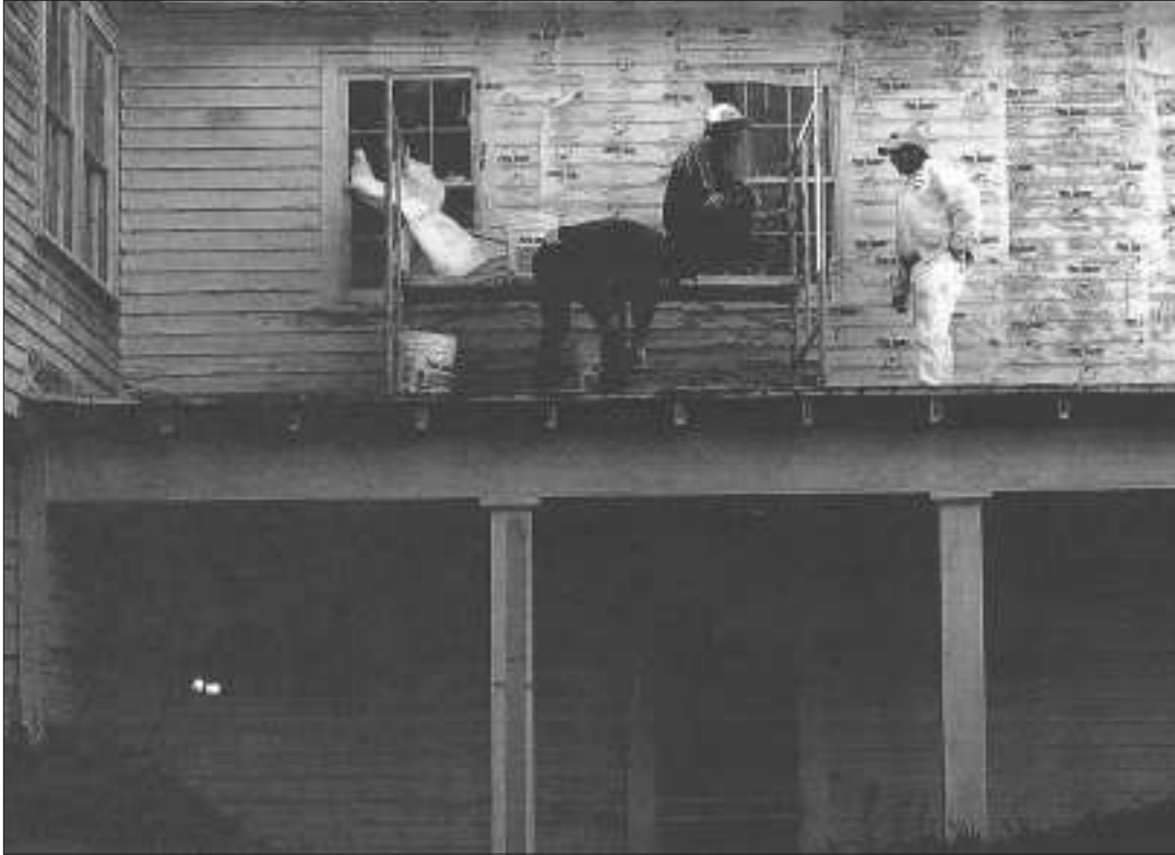
Workers strip paint as part of the restoration of William Faulkner's 160-year-old Rowan Oak home.
