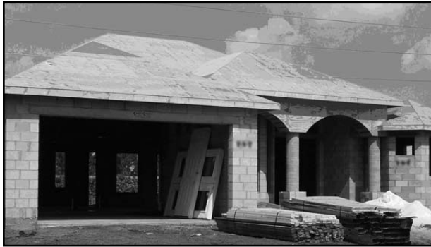
Example of a construction site with building materials and uninstalled doors left unprotected.
