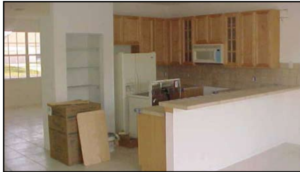
In this house under construction, the front door was left wide open with appliances left uninstalled in the kitchen.
