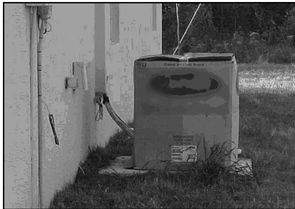
Example of an air conditioning unit delivered and left uninstalled.
