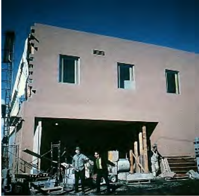
Figure 40. The IRS building in Anchorage, 1964, built using concrete masonry units (source: University of Alaska Anchorage, Consortium Library, Archives & Special Collections, Edith and Edward Lindsay papers, 1964, uaa-hmc-1135-s13).
