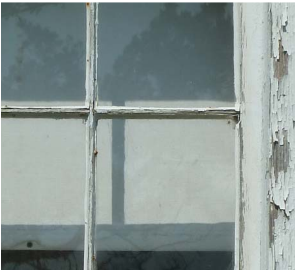
Figure 79. Typical detail showing poor condition of many of the windows.
