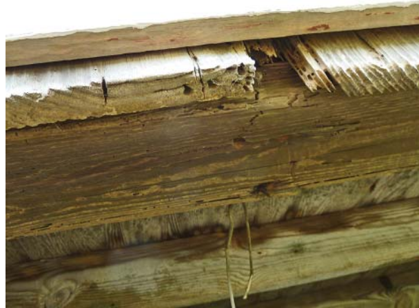
Figure 66. Typical sill and bottom ends of vertical sheathing on the main block of the house.
