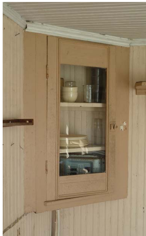
Figure 119. Northwest corner cupboard. The electrical circuit breaker is on the bottom shelf of this cabinet.
