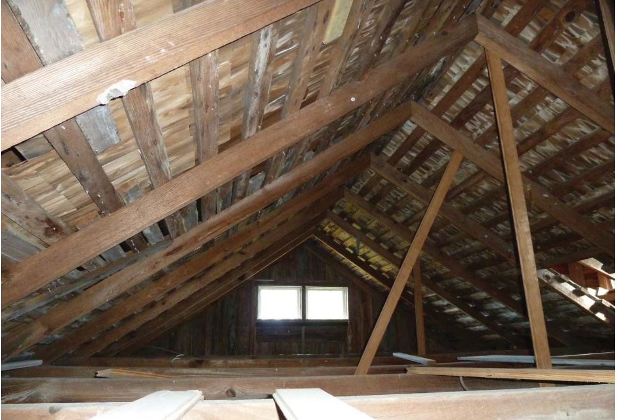
Figure 68. Looking east, showing roof framing and ceiling joists above the main block of the house.
