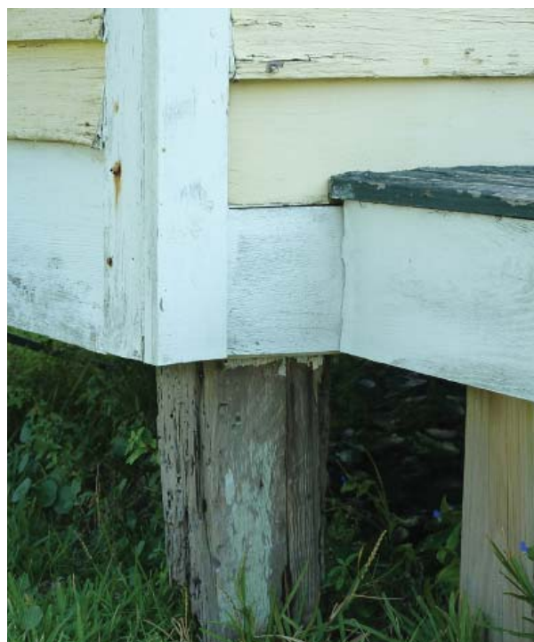
Figure 83. Typical vertical corner boards and the two widths of skirt board found on the house.
