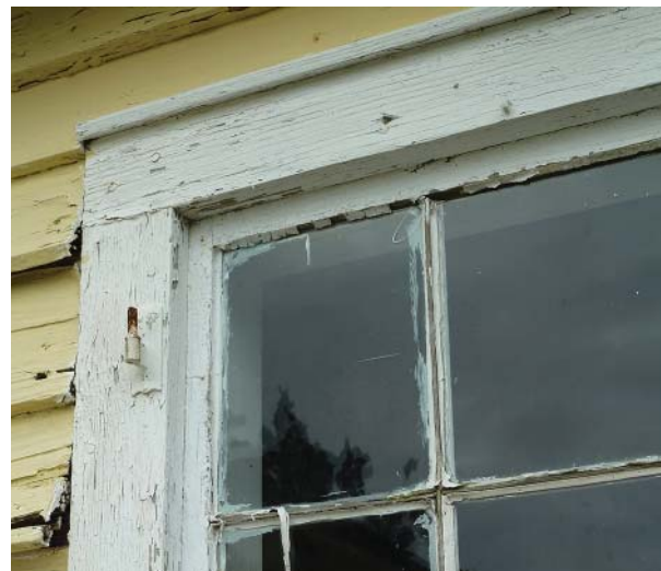
Figure 77. Casing and drip cap typical of all windows, and shutter pintle similar to those found at some older window openings.
