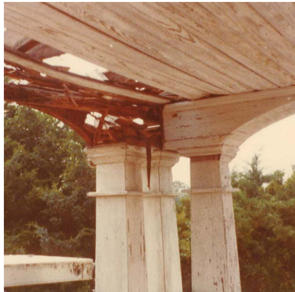
Figure 34. Damage in arches, 1979. (CALO Polaroid album)
