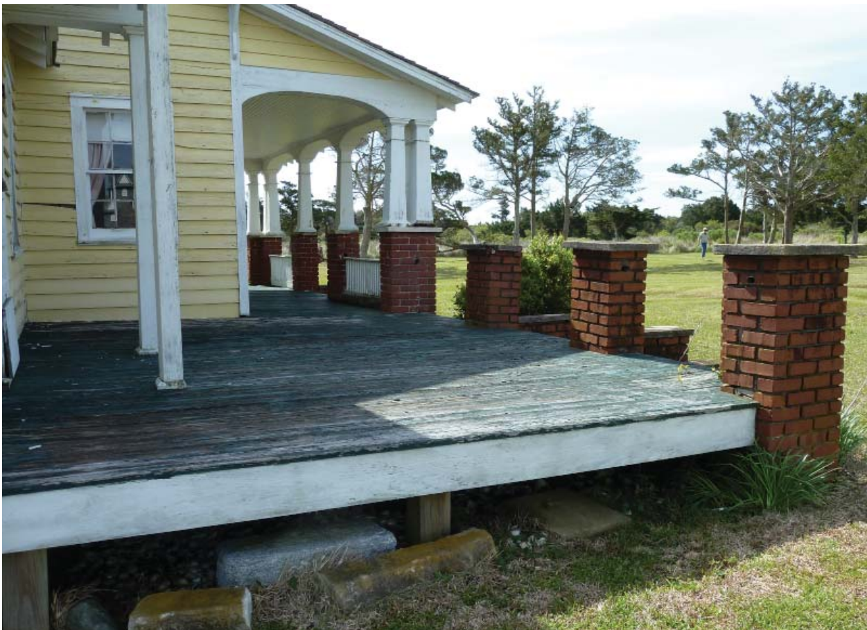
Figure 86. Deck and piers added by Harry Dixon along with the front porch ca. 1928.
