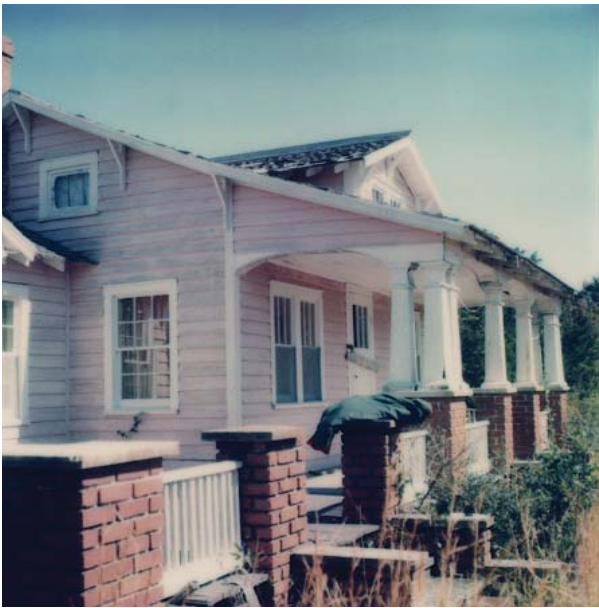
Figure 30. Condition of roof and porch, missing fascia, 1977. (CALO Coll. f79)
