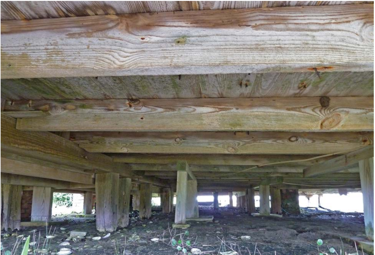
Figure 64. Looking north showing floor framing for the front porch in the foreground.
