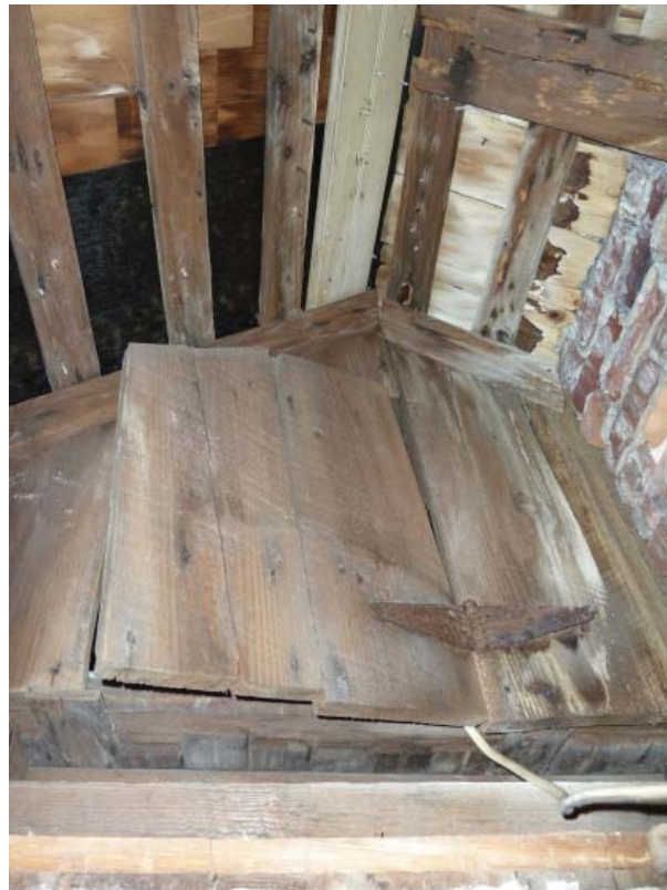
Figure 18. Vertical-board siding of the exterior of the original main block, covered when the west wing was brought up and attached. Shown is a door cut into the siding to lead from attic of wing to attic of main block. (2014 photograph)
