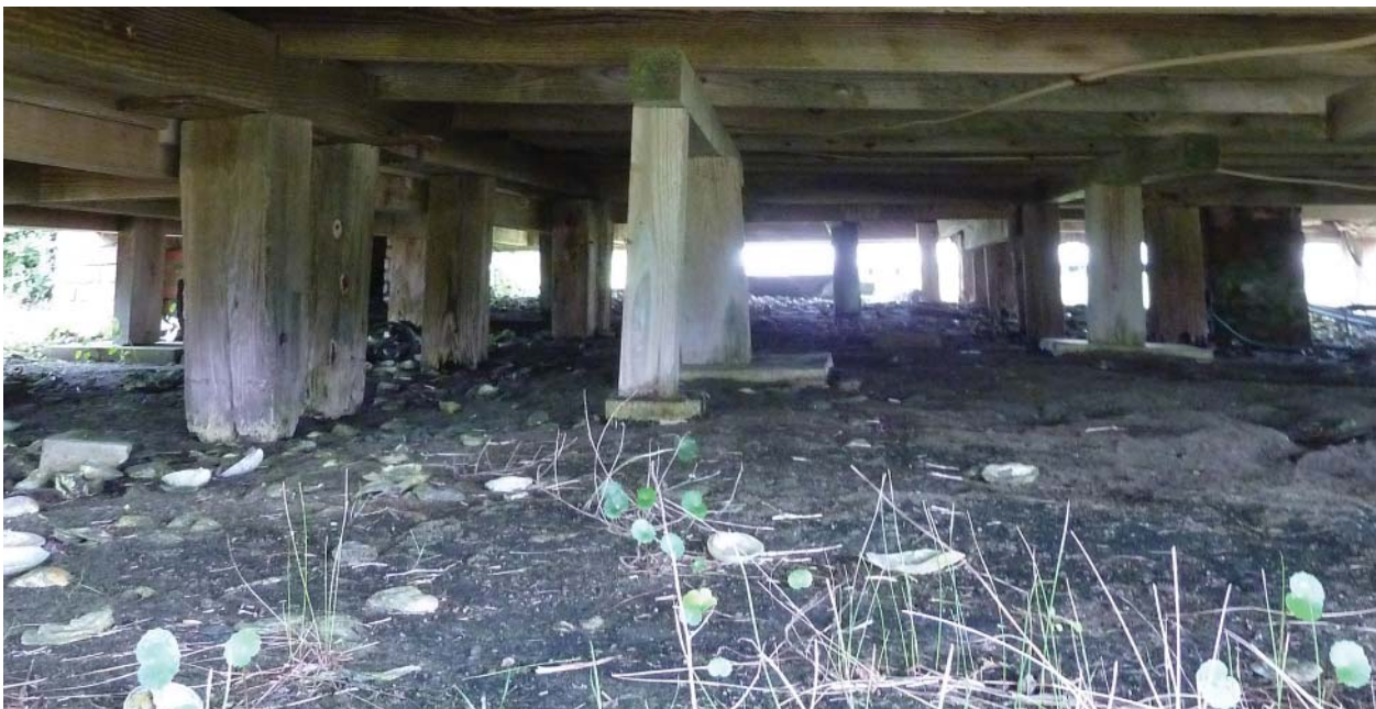
Figure 55. Looking north under west side of front porch and main block, showing historic wood posts at left.
