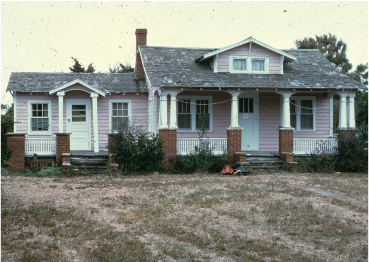
Figure 29. Condition of the house in 1977, also showing the 1960s replacement doors, the 1960s replacement six-over-six sash of the west wing, and the retained Craftsmen-style vertical-pane sash beneath the front porch. (CALO acc. 03355)
