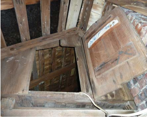
Figure 67. Looking from attic over kitchen wing through door to attic over main block. The white batten on the door has painted lettering from a packing crate that may date to the nineteenth century.
