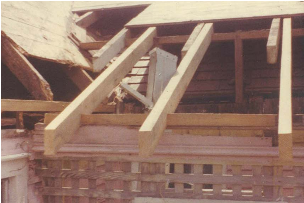
Figure 20. 1979 view showing the rear slope of the Willis roof beneath the higher, longer slope of Harry Dixon's new roof, and the lattice room beneath. The sistered rafters are part of the 1979 repairs. (CALO Polaroid album)
