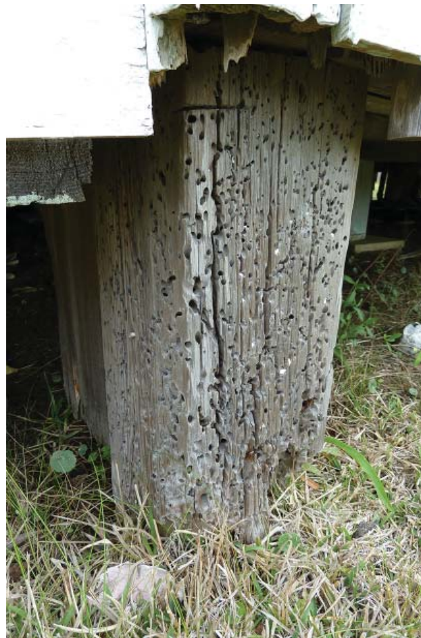
Figure 56. Example foundation post created from salvaged lumber, showing damage characteristic of Teredo navalis , or shipworm. The damage must have occurred prior to the lumber's reuse as a foundation post.
