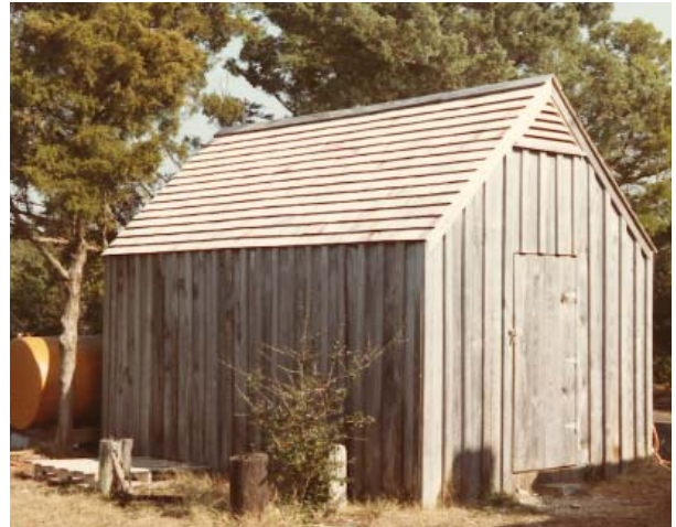
Figure 43. Rebuilt shed with louvered vent in gable end, photographed 1983. (CALO Coll. f295)
