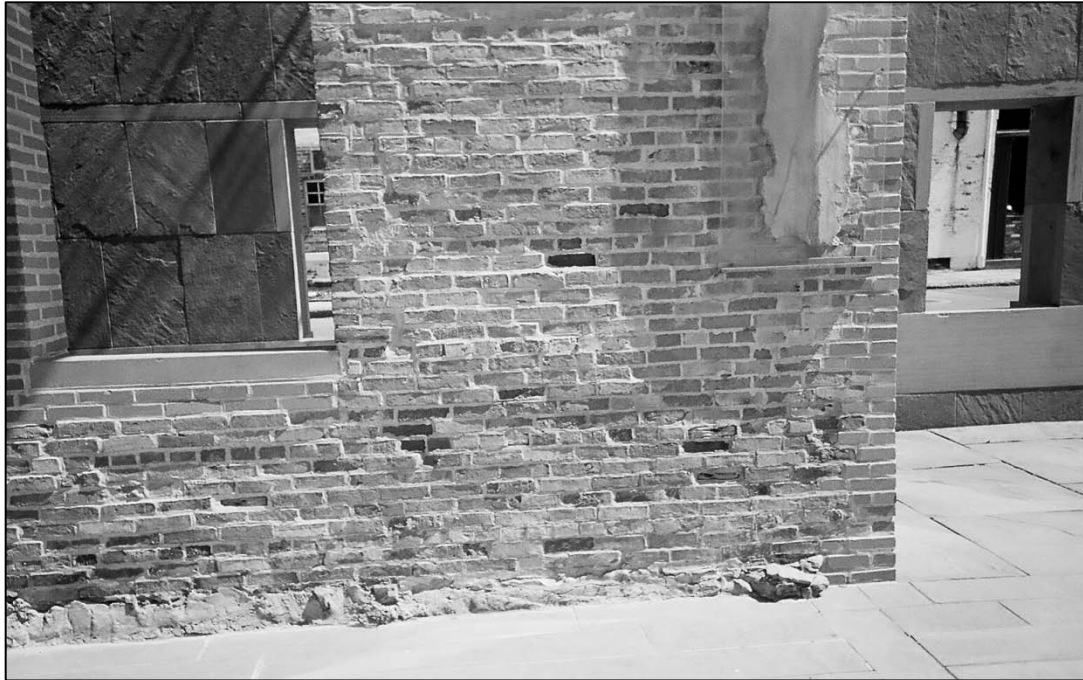
Figure 50. Deterioration along the southeast wall of the Wesleyan Chapel. Courtesy Women’s Rights NHP.
