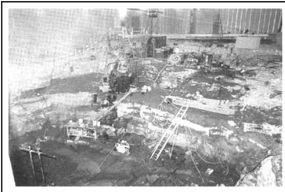
Excavation on the site of JEFF's second theater project, 1990. NPS photo by Al Bilger.
