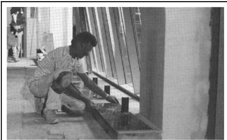
Installation of the marble facing, exterior of the projection booth. NPS photo courtesy Dave Caselli.
