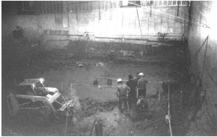
The excavation phase of construction nears completion, 1991. NPS photo by Al Bilger.
