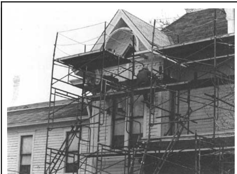
Repairs to the exterior of the Truman site. Courtesy Harry S Truman National Historic Site.
