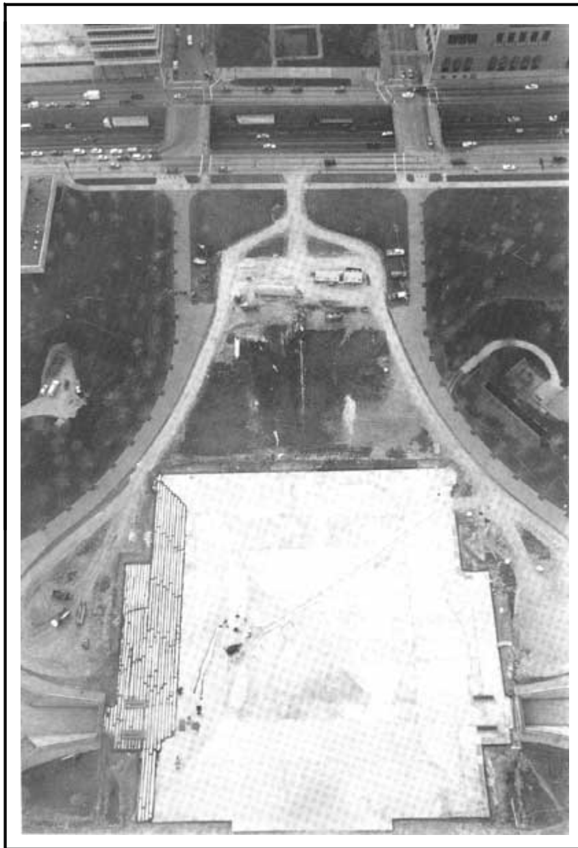
The roof of the underground visitor center/museum exposed for repair, 1990, as seen from the top of the Gateway Arch. NPS photo by Al Bilger.
