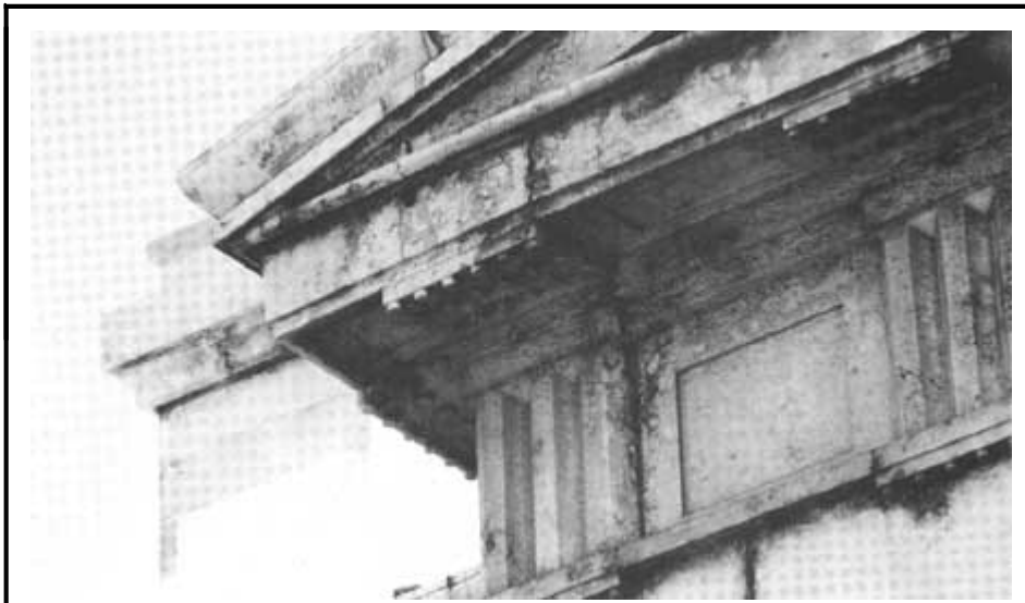
Deteriorated cornice, Old Courthouse, 1978. NPS photo.
