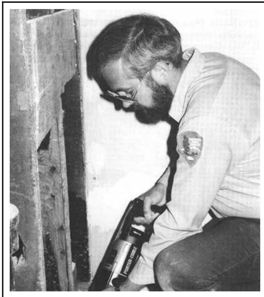
Maintenance Mechanic Lonnie Collins assisting in the construction of an accessible restroom at Ulysses S. Grant, one of many maintenance tasks handled by the HVAC crew. NPS photo by Al Bilger.
