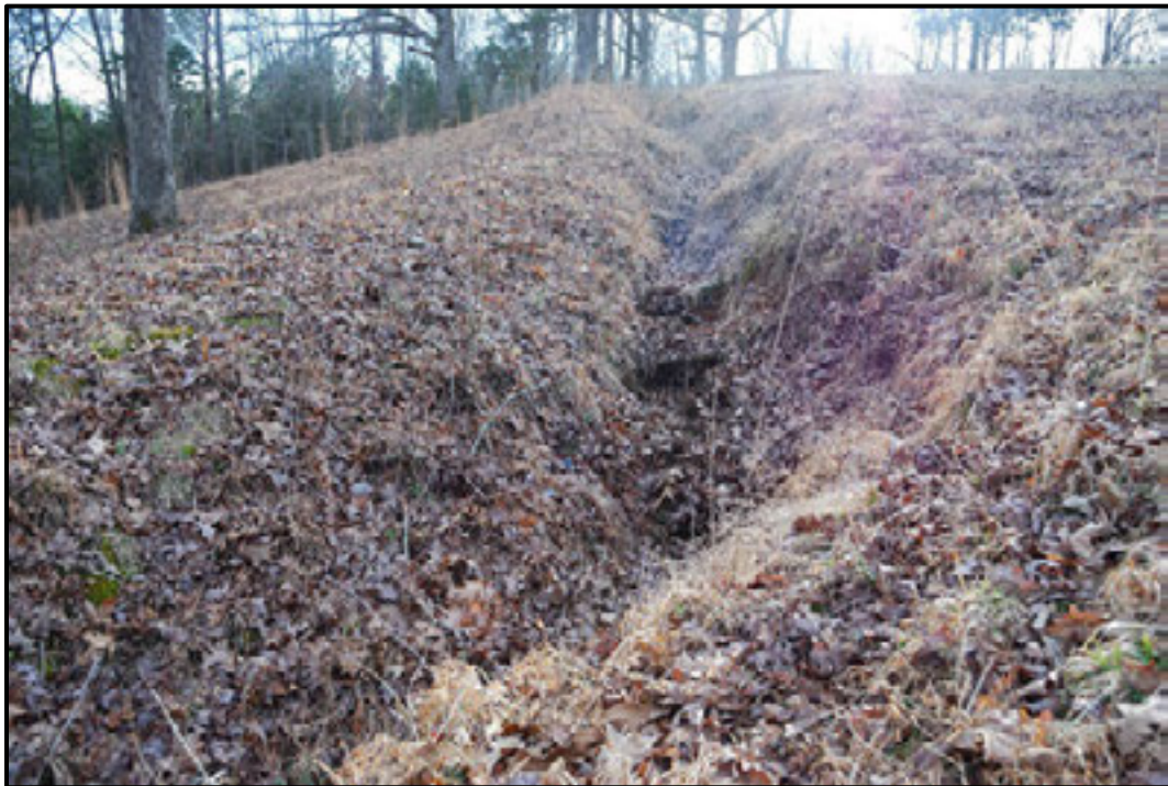
Figure 7.29. Segment 14, erosional damage in the earthwork's ditch.
