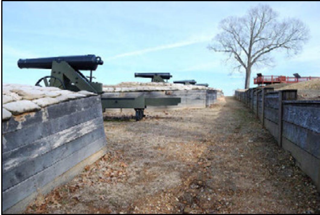
Figure 7.10. View from pedestrian access to guns; note damage from runoff.
