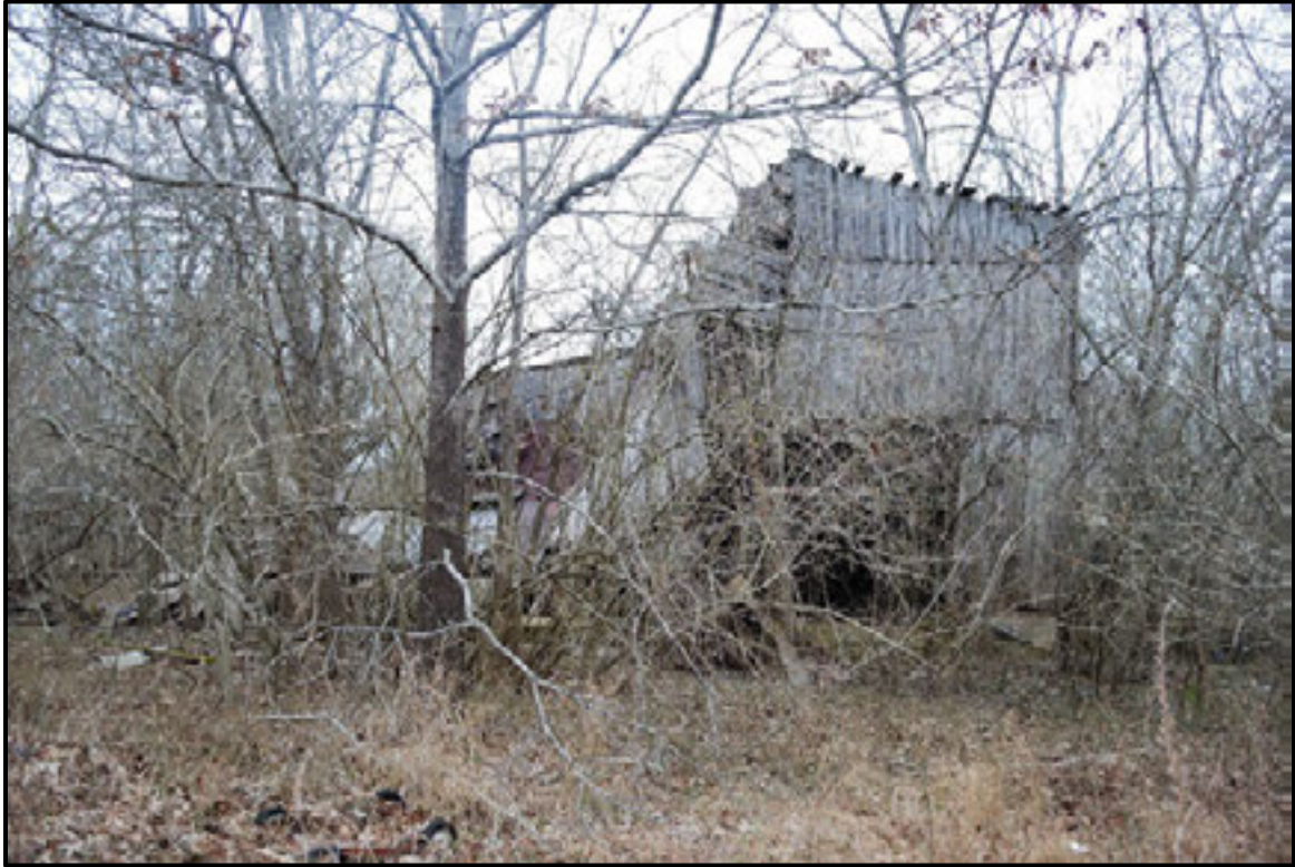
Figure 7.139. South elevation of collapsing barn (Resource E).
