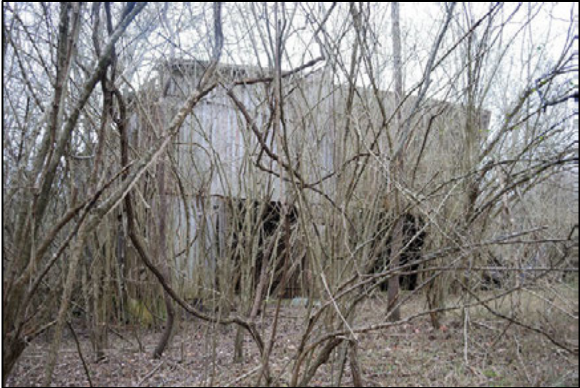
Figure 7.140. North elevation of collapsing barn (Resource E).
