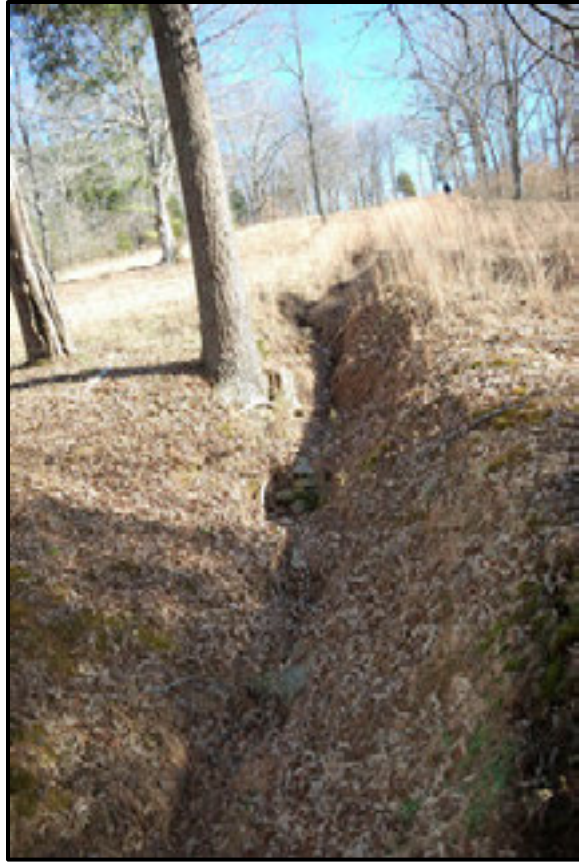
Figure 7.33. Segment 16, water damage to ditch on western slope of hill.
