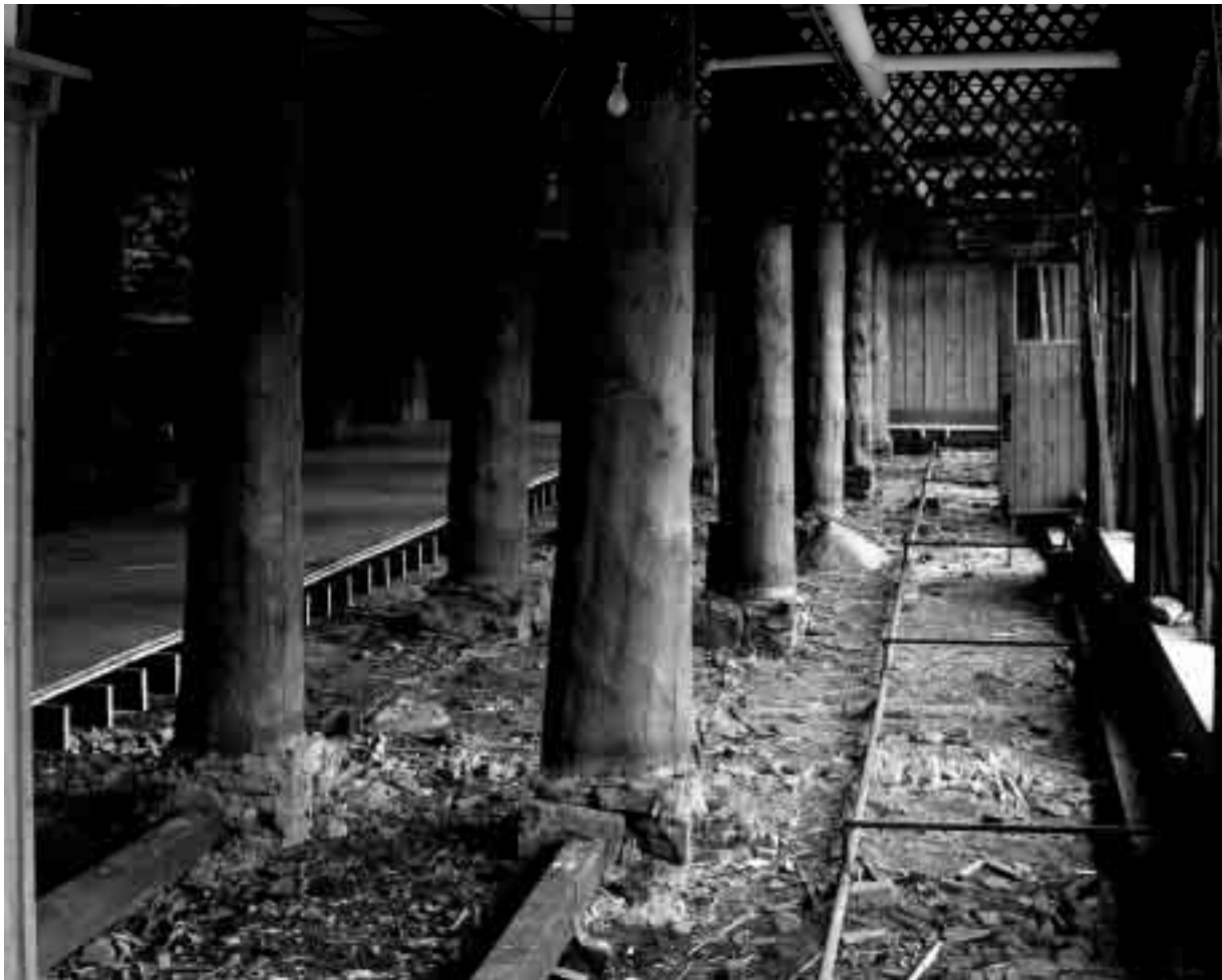
Base of original log columns set in main building. The typical peeled log column measured approximately 36 inches at its base and reduced to approximately 30 inches at its peak. This photo shows the floor of the Grill Room opened for repair work to bad concrete bases under log columns in 1952. Courtesy Glacier National Park Archives
