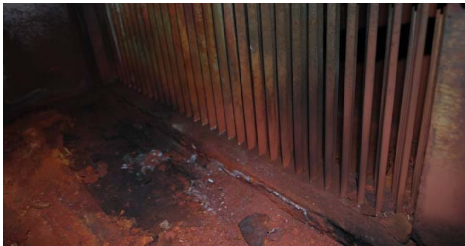
Photograph 10 - DG5 air cooler, outlet area
