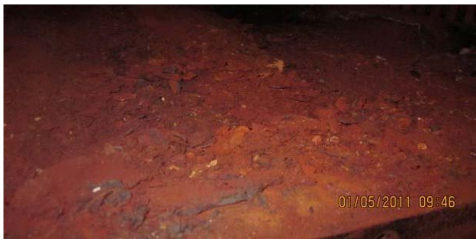
Photograph 9 - DG5 air cooler, outlet area
