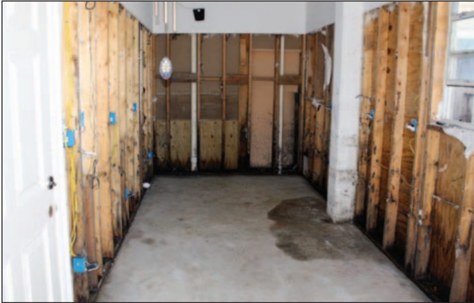
Figure 3-23: Enclosed area that was not finished with flood-resistant materials, nor did it have flood openings (Plaquemines Parish, LA).
