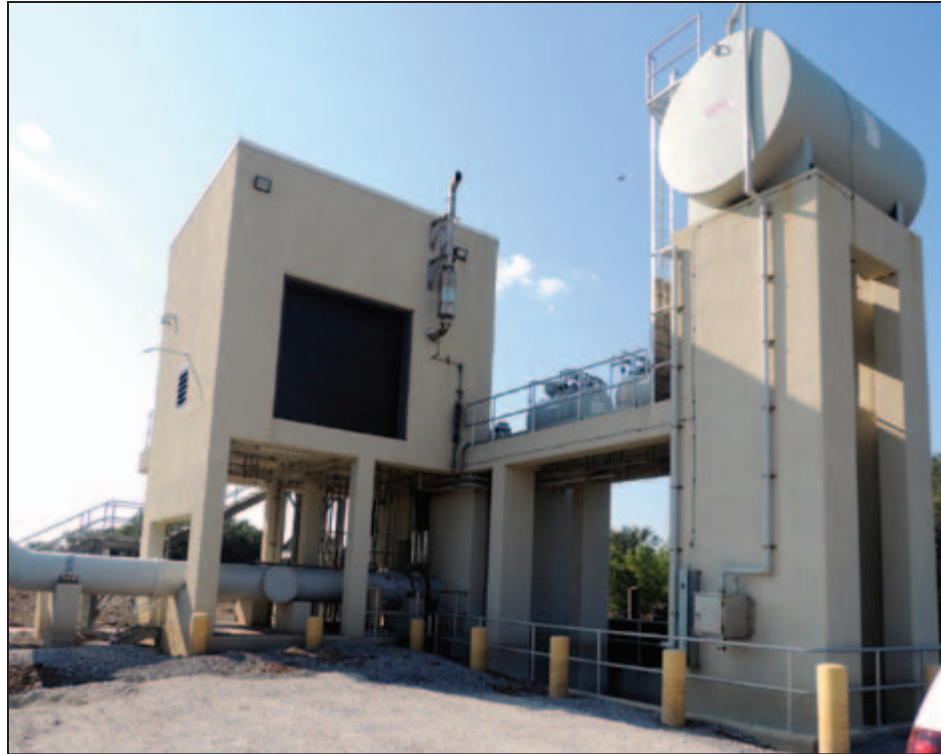
Figure 4-20: Elevated stormwater pump station south of Braithwaite Park reconstructed after Hurricane Katrina with FEMA Public Assistance funds (Braithwaite [East Bank] – Plaquemines Parish, LA).
