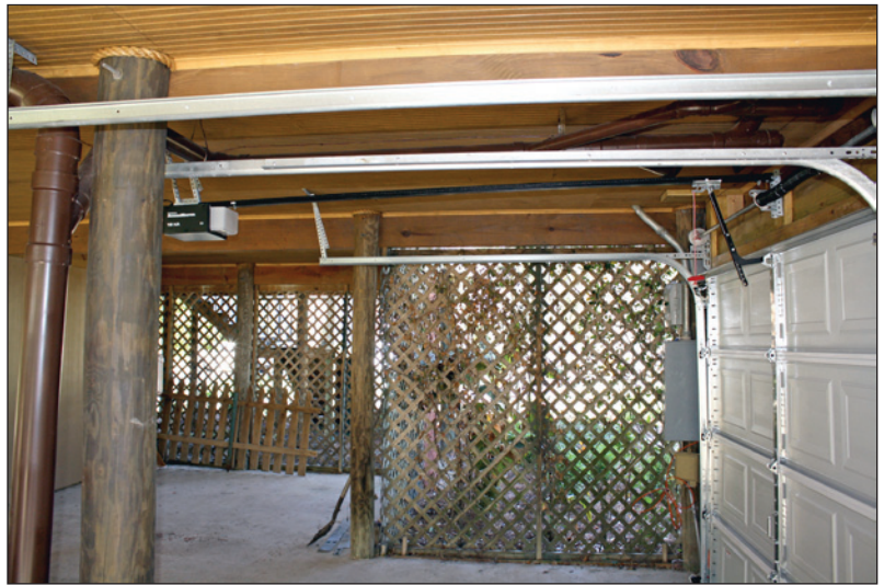
Figure 2. Space under an elevated building used as a parking area (St. Tammany Parish, LA, Hurricane Isaac)
