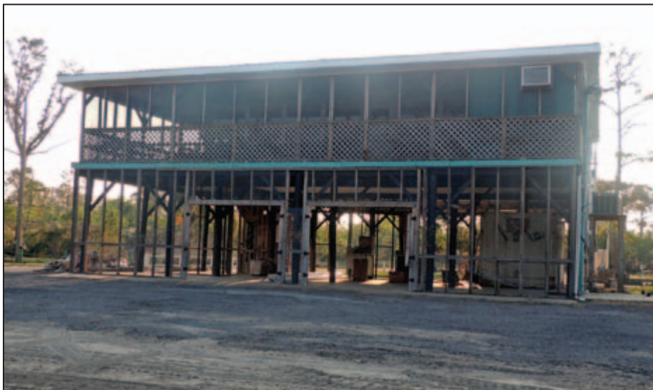
Figure 5-24: Nonresidential structure with damage to the screen surrounding the area under the lowest floor (Structure A in Figure 5-18) (St. John the Baptist Parish, LA).
