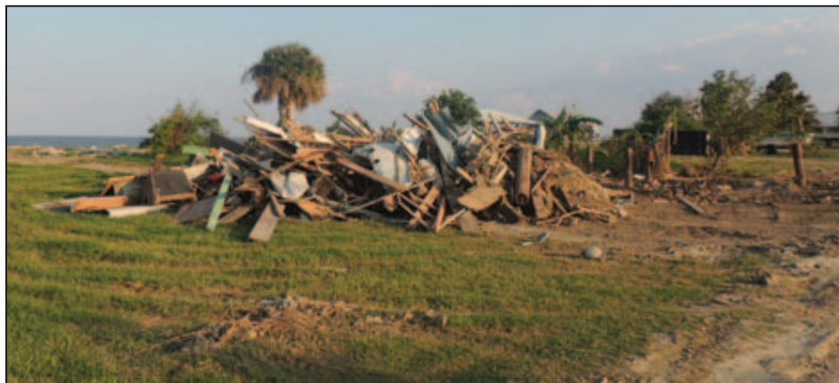
Figure 5-22: Debris pile of waterfront single-family residence along the west bank of Lake Pontchartrain (Structure D in Figure 5-18) (St. John the Baptist Parish, LA).
