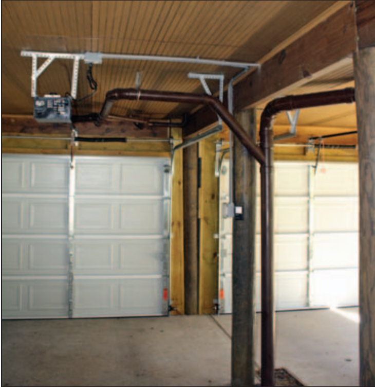
Figure 3-25: Elevated house with combustible materials and vehicle parking below elevated space (Mandeville, LA).
