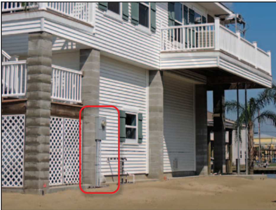
Figure 3-17: Electric meter attached to foundation pier (Plaquemines Parish, LA).
