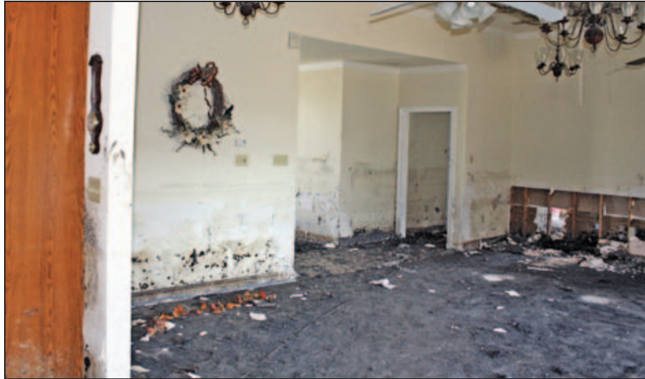
Figure 5-7: Interior damage to the non-elevated residence (Plaquemines Parish, LA).
