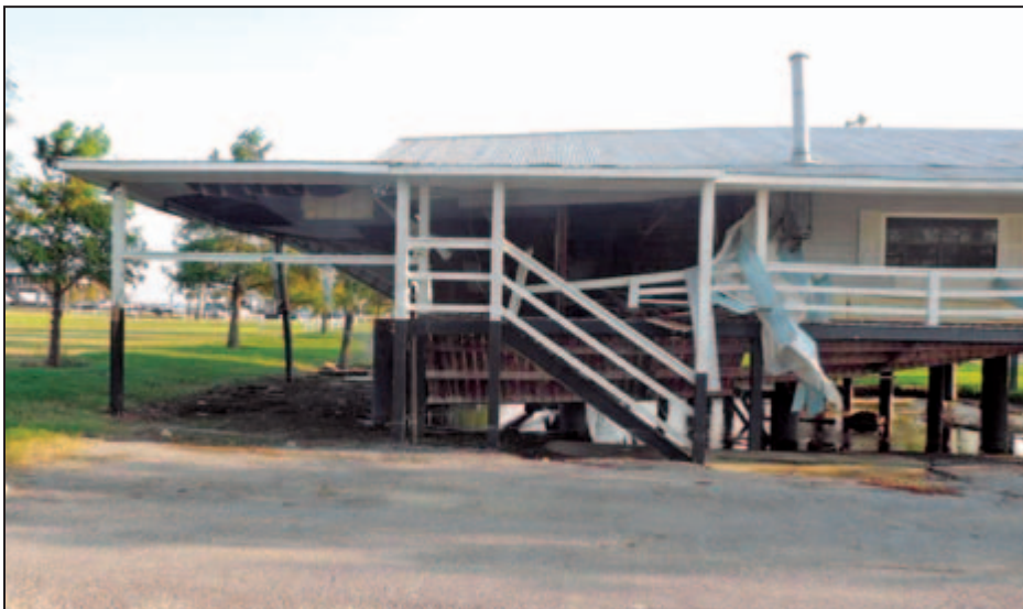
Figure 5-19: Surge damage to lakefront residential structure (Structure B in Figure 5-18) (St. John the Baptist Parish, LA).
