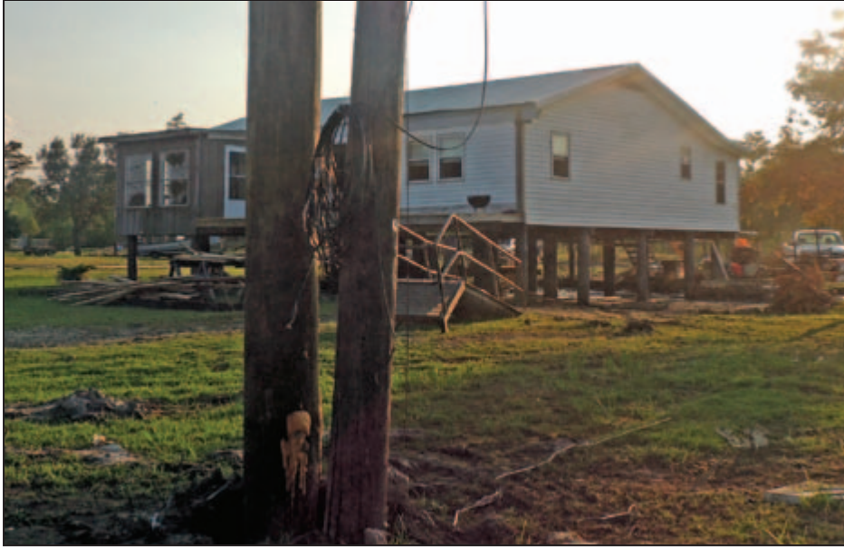
Figure 5-23: Residential building elevated approximately 3 to 4 feet above grade that lost stairs and received other damage below the lowest floor (Structure C in Figure 5-18) (St. John the Baptist Parish, LA).
