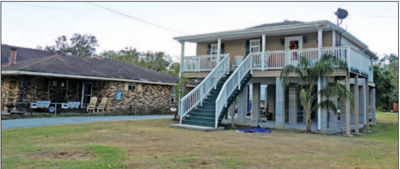
Figure 3-2: Damage was observed in most at-grade slab foundation residences, while minimal damage was observed in adjacent elevated properties (Barataria, LA).
