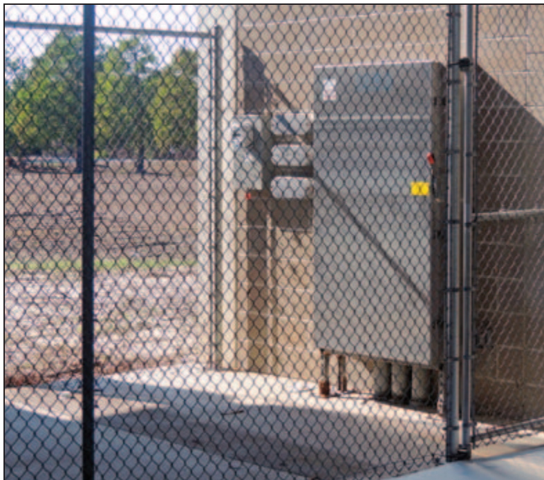
Figure 4-6: The Braithwaite Auditorium generator transfer switch and other electrical components were built at grade and damaged by floodwaters (Braithwaite Park [East Bank] – Plaquemines Parish, LA).
