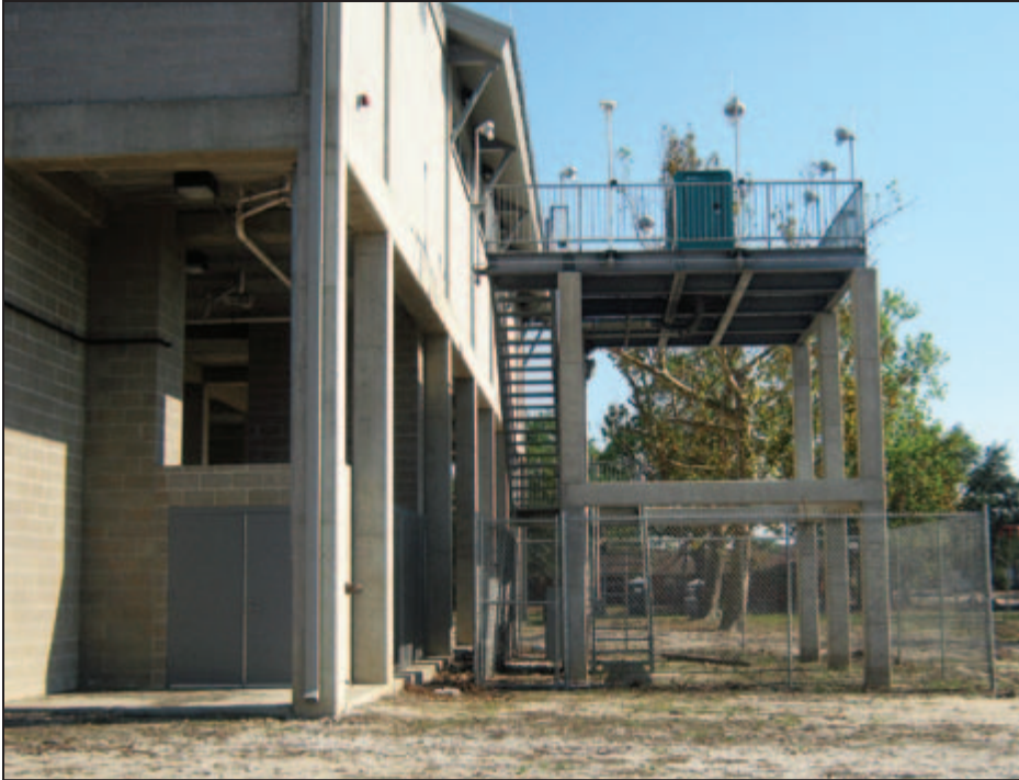
Figure 4-3: The Braithwaite Auditorium has an elevated generator for emergency power (Braithwaite Park [East Bank] – Plaquemines Parish, LA).
