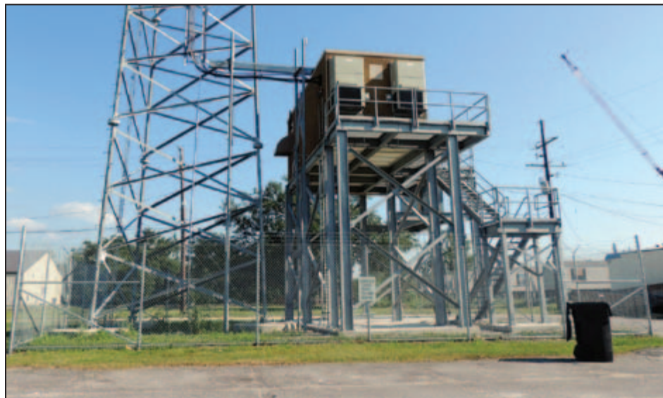
Figure 4-18: Cellular tower equipment on elevated platform near Port Sulphur Community Center (Port Sulphur [West Bank] – Plaquemines Parish, LA).
