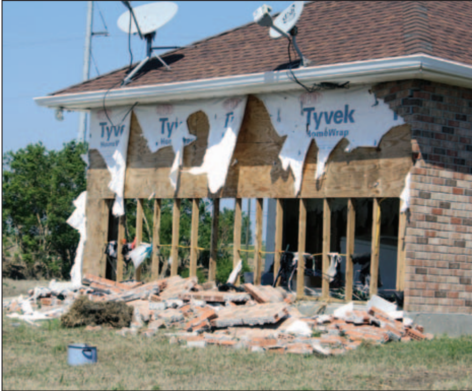
Figure 5-5: Exterior damage to the garage of the non-elevated residence (Plaquemines Parish, LA).
