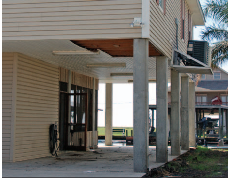
Figure 3-24: Loss of the sheathing from the underside of an elevated building due to wind gusts (reported to exceed 80 mph) that exceeded the capacity of the vinyl siding (Plaquemines Parish, LA).
