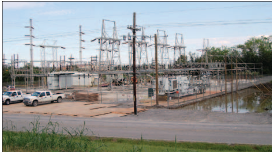
Figure 4-13: Electrical repairs being completed after substation equipment was inundated by floodwaters (Braithwaite [East Bank] – Plaquemines Parish, LA).
