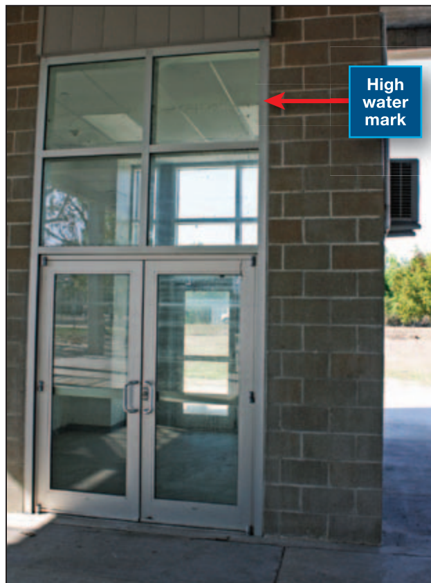
Figure 4-2: HWM visible on glass at entrance to elevators below lowest floor of Braithwaite Auditorium (Braithwaite Park [East Bank] – Plaquemines Parish, LA).
