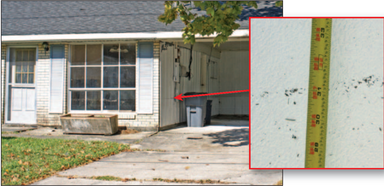
Figure 3-3: Typical flood depth of at-grade slab foundation residences; inset illustrates flood depth of 31 inches above the at-grade slab foundation (Slidell, LA).
