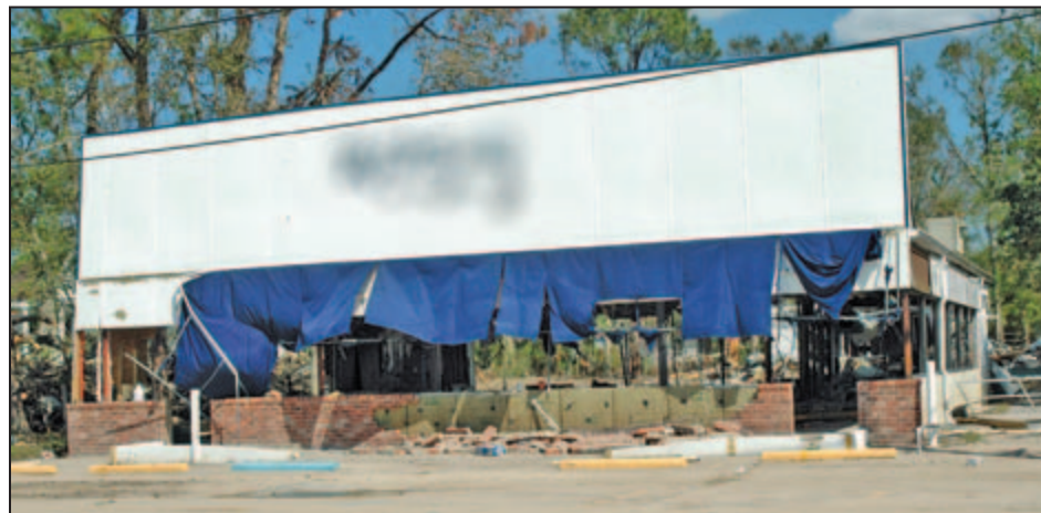
Figure 5-11: A nonresidential building on Lakeshore Drive in Mandeville post-Hurricane Katrina (Mandeville, LA).
