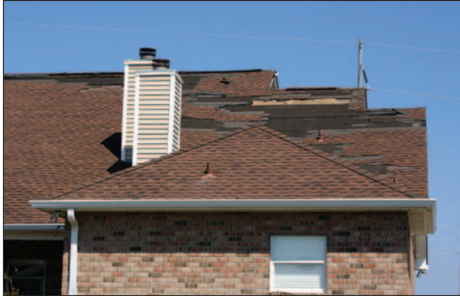
Figure 5-3: Roof cover loss at non-elevated residential building (Plaquemines Parish, LA).
