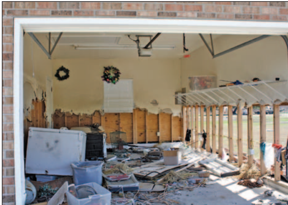
Figure 5-4: Interior damage to the garage of the non-elevated residence (Plaquemines Parish, LA).
