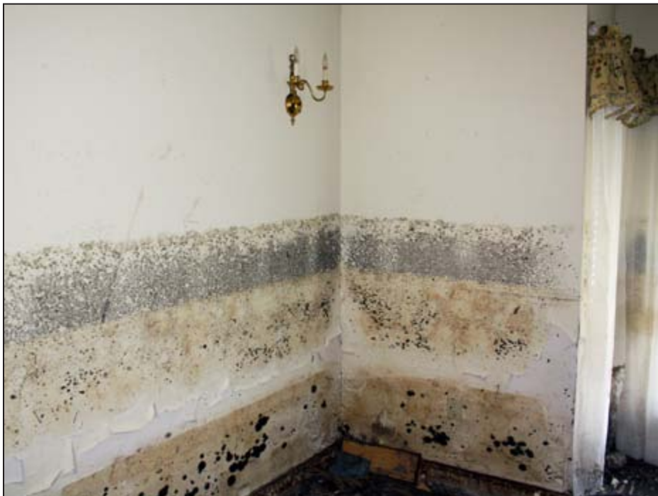
Figure 5-6: Interior damage to the non-elevated residence (Plaquemines Parish, LA).
