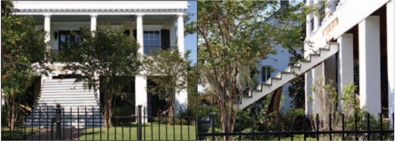
Figure 3-20: Front and side view of stair damage to elevated waterfront residential building due to closed riser, inadequate foot anchoring, and insufficient connection with the building frame (Mandeville, LA).
