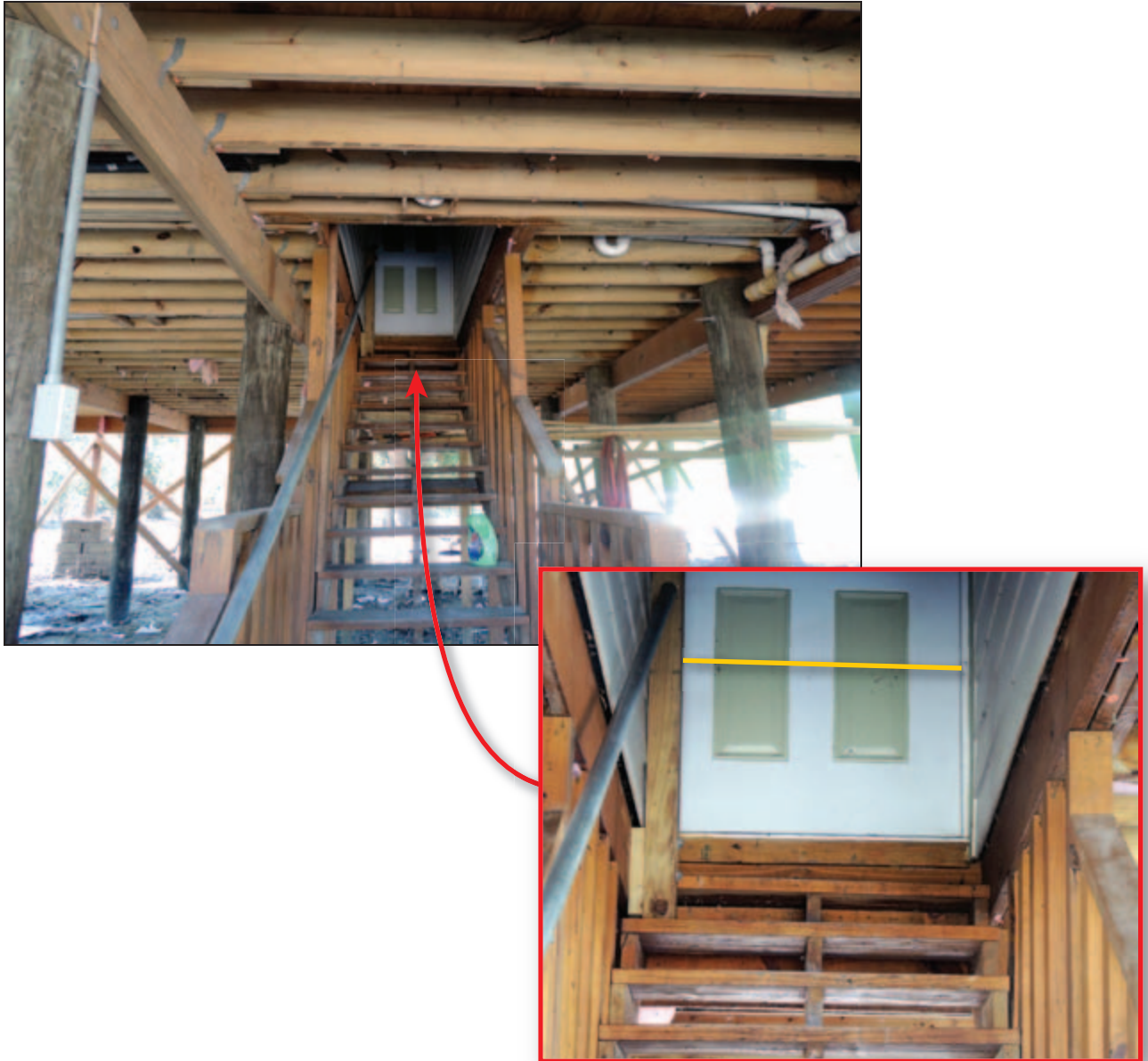
Figure 5-16: Elevated house built in 2009 on Highway 39 had approximately 2 feet of water infiltrate the first floor; inset: yellow line illustrates observed HWM on door (Plaquemines Parish, LA).
