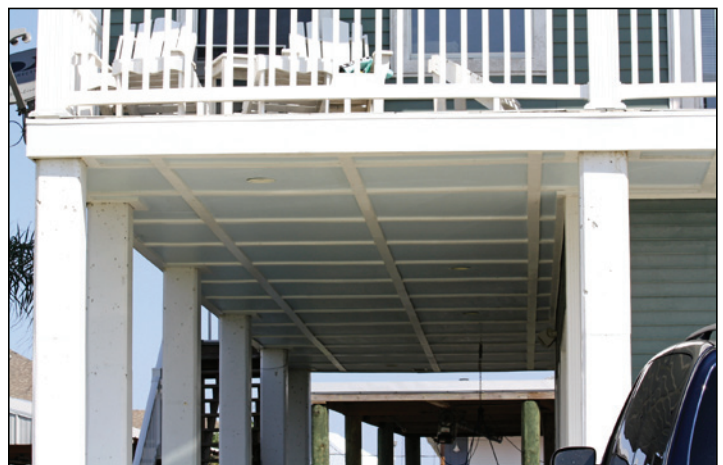
Figure 4. Wood sheathing under a house near the one shown in Figure 3 did not fail; this is not a fire-resistant-rated assembly (Plaquemines Parish, LA, Hurricane Isaac)
