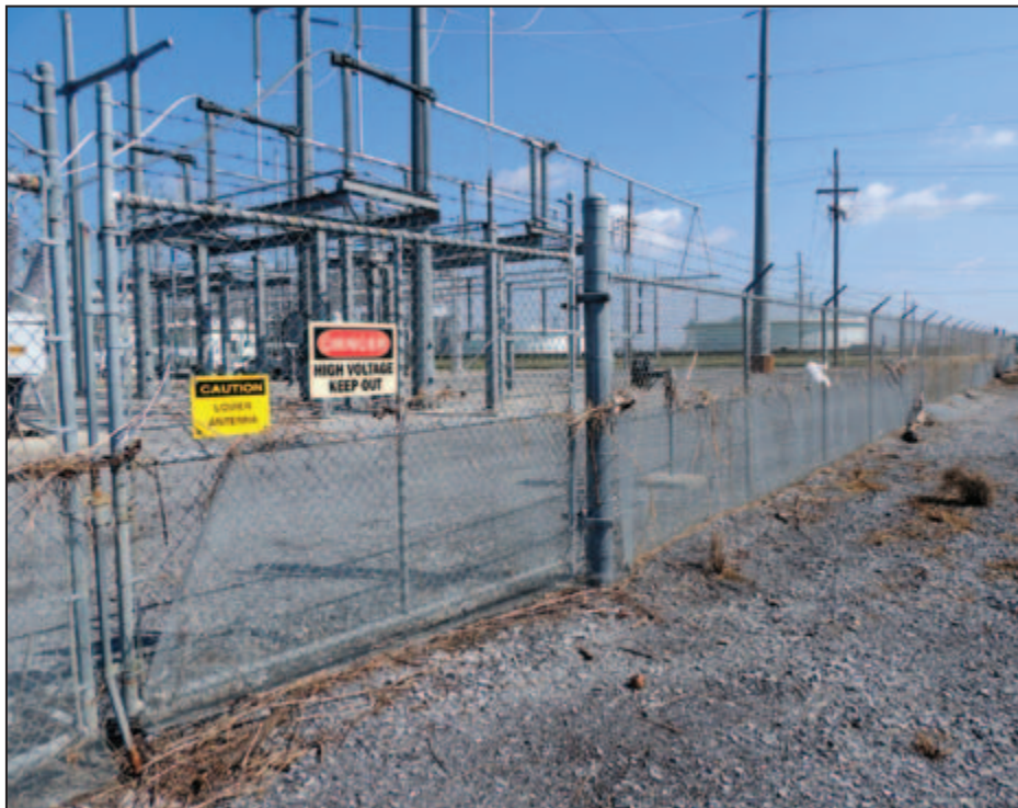
Figure 4-16: Flood inundation depths were 4 to 5 feet above grade at the substation protected by the berm that was overtopped (Belle Chase [West Bank] – Plaquemines Parish, LA).
