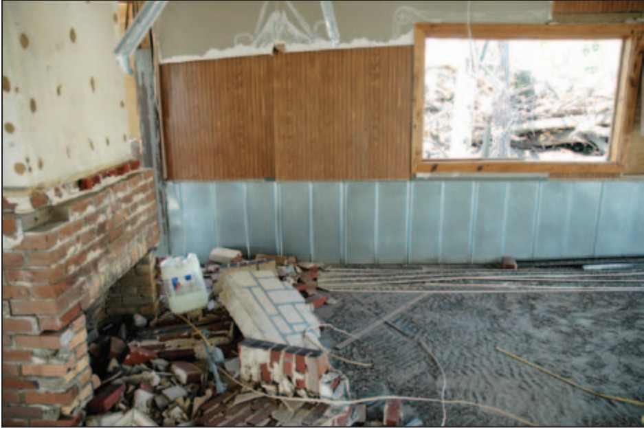
Figure 5-13: Interior damage from Hurricane Katrina to nonresidential building on Lakeshore Drive (Mandeville, LA).
