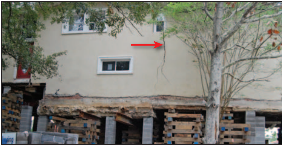
Figure 3-11: Slab-on-grade elevation with structural cracks due to differential lifting (Slidell, LA).
