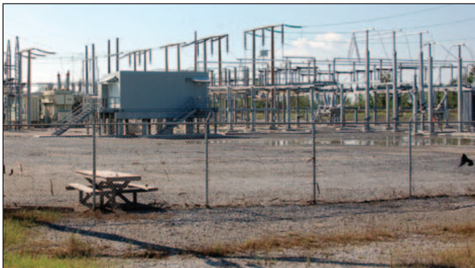
Figure 4-14: Substation equipment elevated several feet above grade (Belle Chase [West Bank] – Plaquemines Parish, LA).
