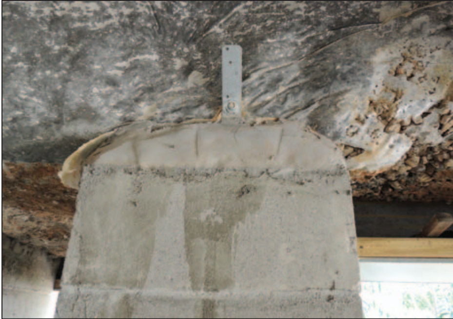
Figure 3-14: Structurally insufficient connection to pier. This house had a total of 7 such connections out of 17 piers supporting the structure (Mandeville, LA).
