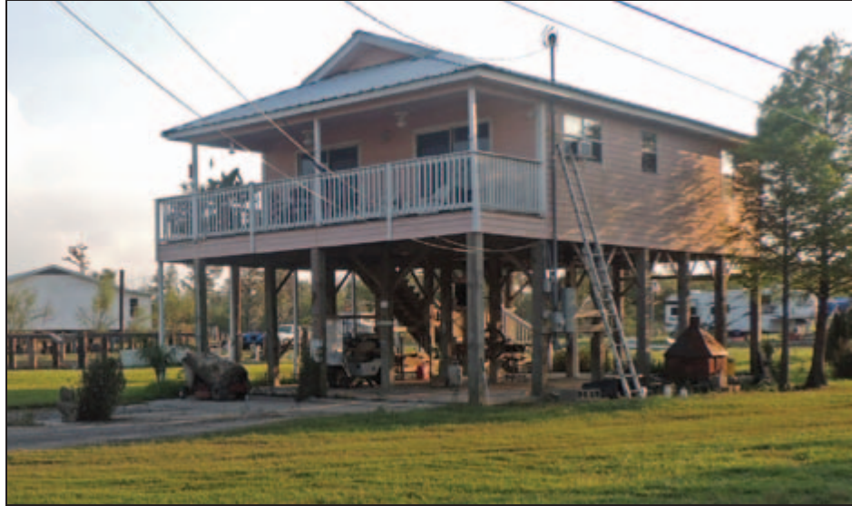
Figure 5-20: Elevated residence with no observed damage (Structure E in Figure 5-18) (St. John the Baptist Parish, LA).
