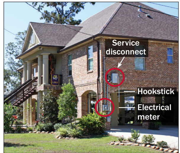
Figure 4. Other than the electrical meter, all the electrical components are elevated and protected from flooding at this home. The system incorporates an electrical service disconnect that is remotely operable with a hookstick (St. Tammany Parish, LA).
