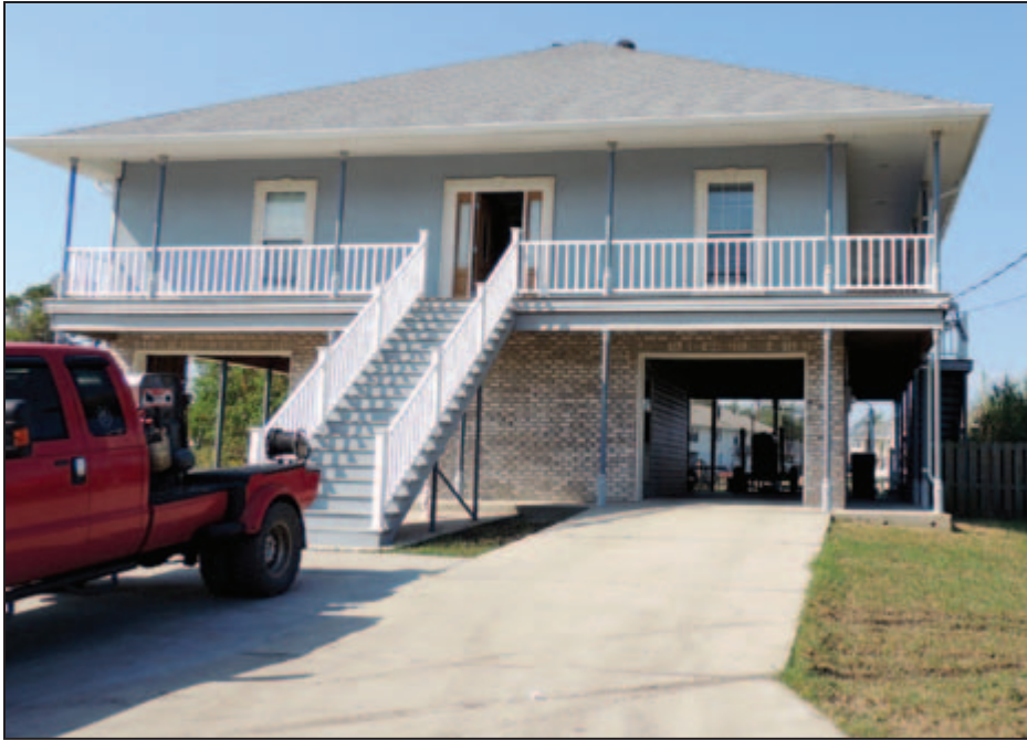
Figure 3-5: Minimal damage was observed in most elevated residences. The USGS HWM near this location was 9.74 feet, compared to an effective BFE of Zone A14 (EL12), Katrina ABFE of Zone AE (EL13), and preliminary FIRM of Zone VE (EL16) (Orleans Parish, LA).
