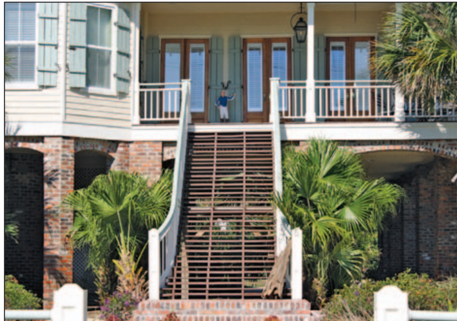
Figure 6-1: Residential stairs with partially open risers to reduce potential flood damage (Mandeville, LA).
