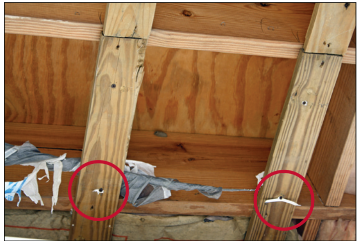
Figure 3. Covering under an elevated building was lost when the vinyl soffit paneling tore around fastener heads during high winds (Plaquemines Parish, LA, Hurricane Isaac)
