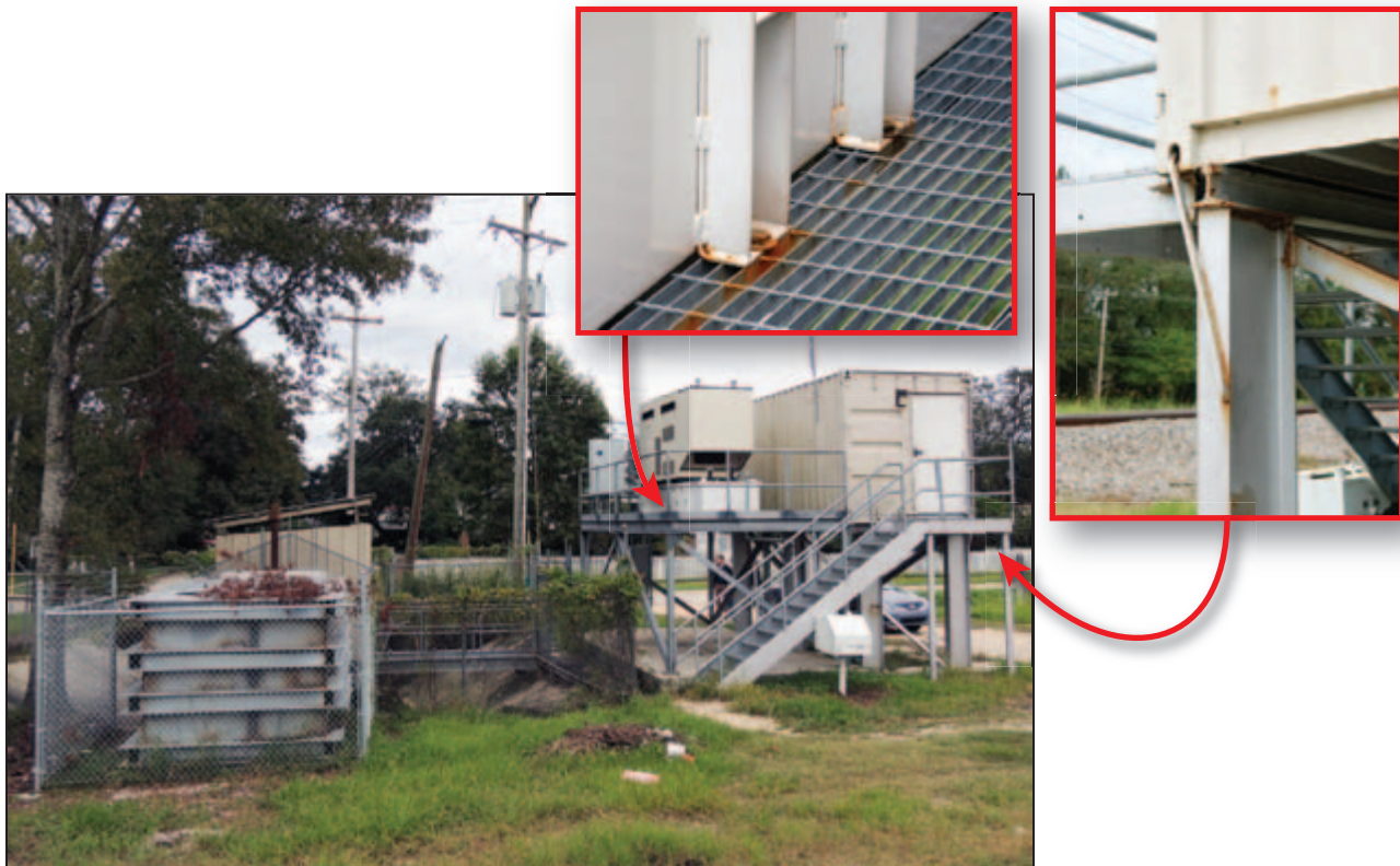
Figure 4-21: The control panels and generator at this pump station were elevated as part of a mitigation measure with FEMA Public Assistance funds; insets illustrate connections between equipment and platform (Slidell, LA).
