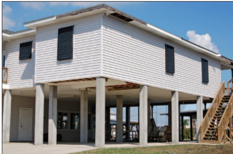
Figure 3-7: Roof soffit and fascia damage to Exposure C residential building (Plaquemines Parish, LA).
