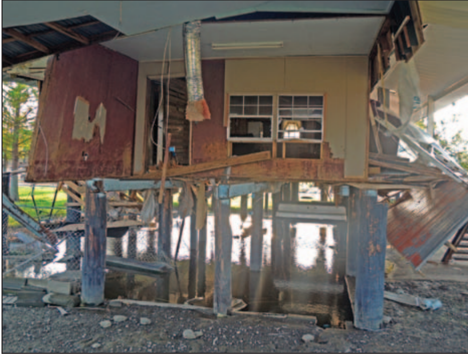
Figure 3-1: Wave and surge damage to a residential building. The house is located in Zone V along Lake Pontchartrain's western shoreline (Saint John the Baptist Parish, LA).
