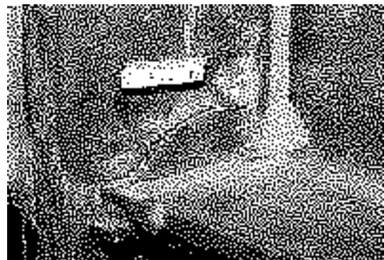
b. Column Flange "Divot" Fracture
