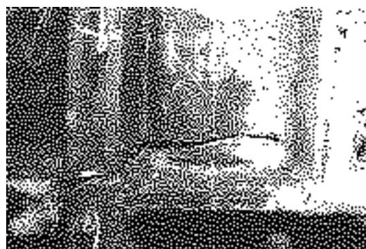
b. Fracture Progresses into Column Web
