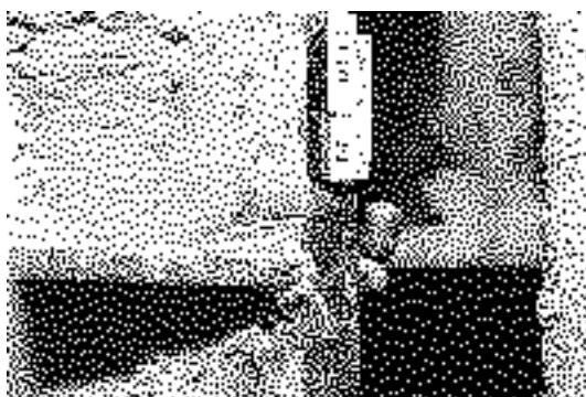
a. Fractures through Column Flange
