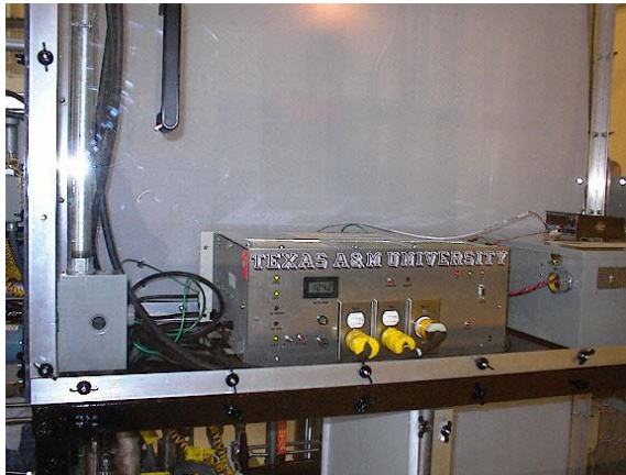
Figure 8-40a. Texas A&M Inverter operating on DOE NETL Fuel Cell on August 14, 2001
