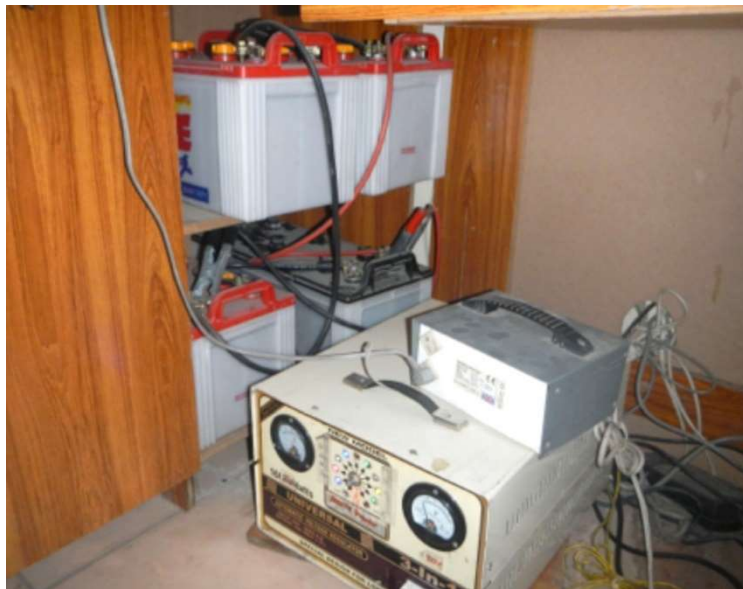
Picture 40: Homemade power conditioner and uninterruptible power supply for an ultrasound machine and clinical computers
