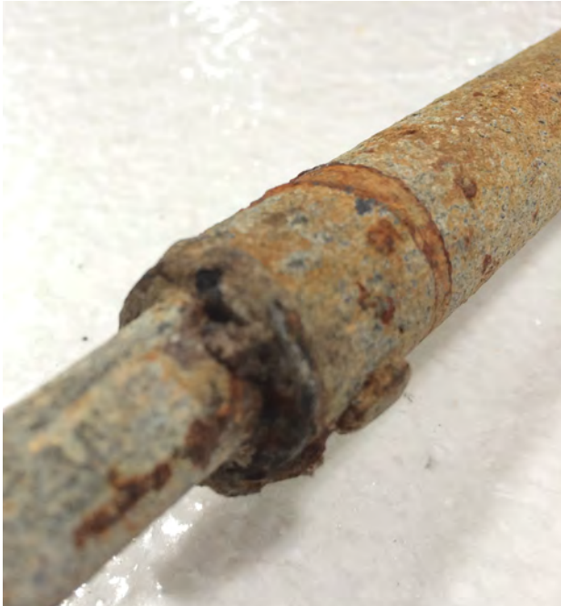
Figure 15.3. Photograph of the joint shows a band of rust indicating the position of a possible clamp or bracket. (Photo by Michael Scafuri, courtesy of FOTH)
