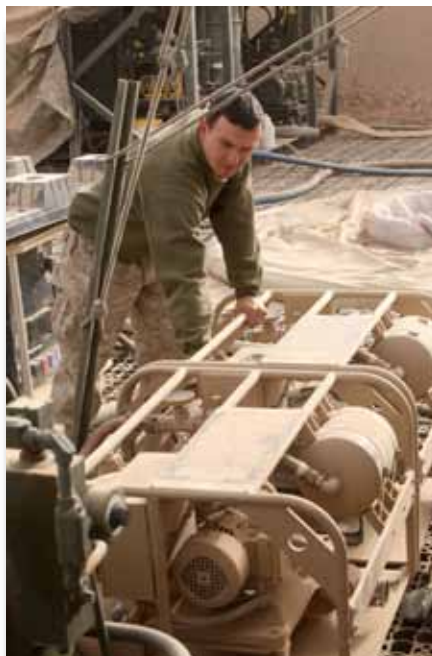
Lance Cpl. Andrew C. Grencer, a water purification technician with Utilities Platoon, Service Company, 8th Engineer Support Battalion, 1st Marine Logistics Group (Forward), turns on a water pump at Forward Operating Base Nolay in Helmand province, Afghanistan, Dec. 5, 2010. Water purification technicians with 8th ESB provide laundry and shower services for Marines with 3rd Battalion, 5th Marine Regiment, 1st Marine Division (Forward), who operate from the FOB. Photo: Lance Cpl. Kenneth C. Jasik
