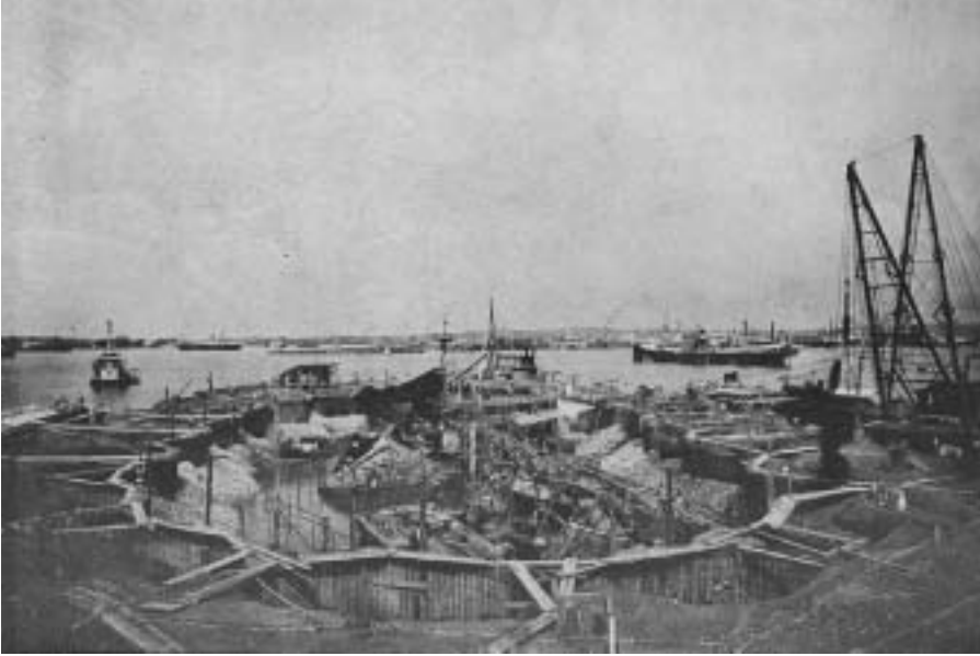
Earth-filled cofferdams 54 feet in diameter provide access to the wreck of the battleship Maine on the bottom of Havana harbor.
