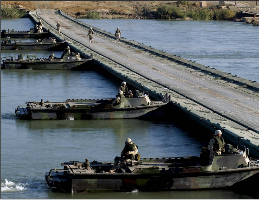
Figure 10.3. Bridge erection boats (BEBs) employed to stabilize an improved ribbon bridge (IRB) during training exercises. Courtesy of US Army.
