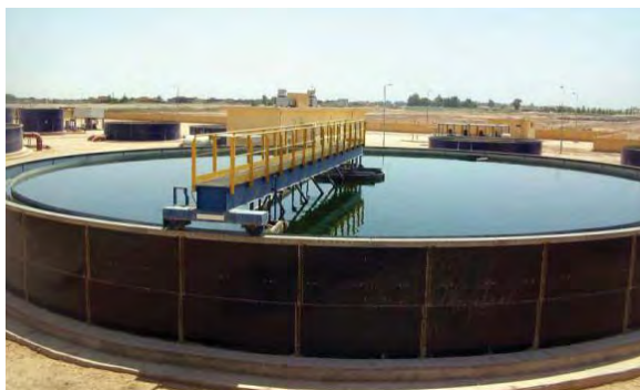
Corps-constructed and designed treatment system in Fallujah
