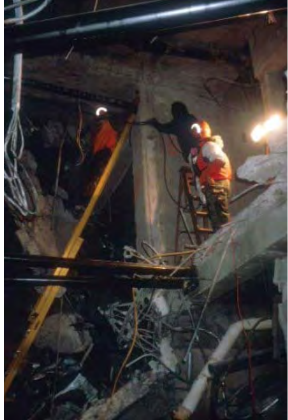
St. Louis District Structure Specialist Tom Niedernhofer conducting inspection at Oklahoma City bombing site
