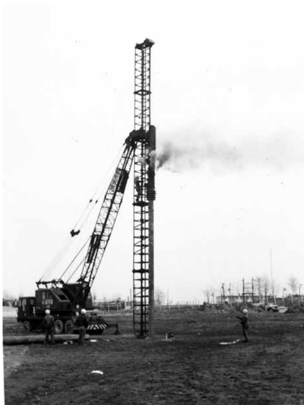
Workers using a pile driving machine during construction of troop housing at Camp Humphreys in the 1970s.
