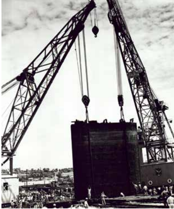
At Incheon, one of the giant leaves of the miter gate is hoisted for repair, November 1959. Credit: Photo by Sergeant Ray Boswell, FED, PAO-FED Historical Files
