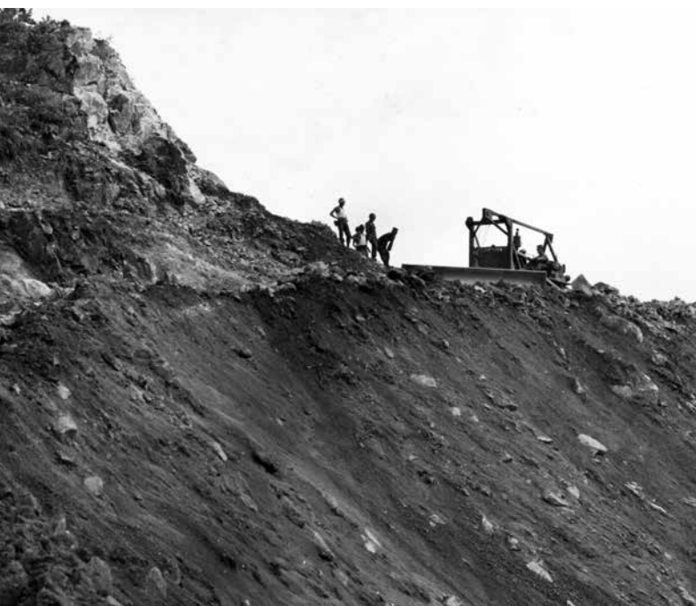
Workers inspect progress during construction of a road to a Hawk or Nike missile site.
