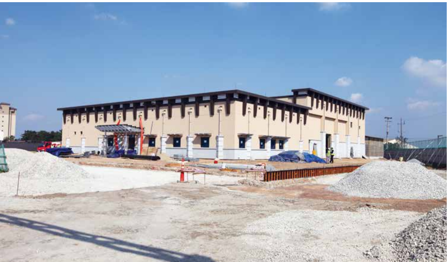
FED works to complete a new flight simulator facility for the U.S. Air Force at Kunsan Air Base, 2012.
