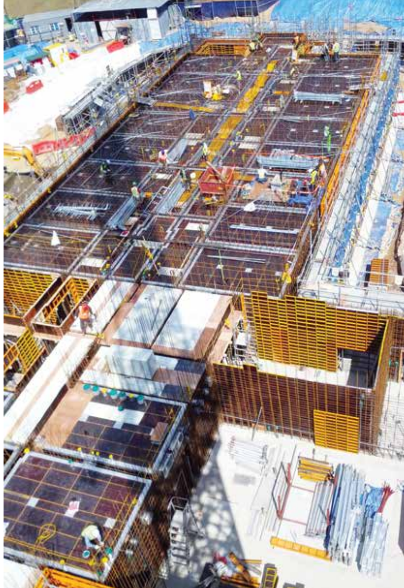
Construction of barracks at Camp Carroll using a new down slab system, 2014.
