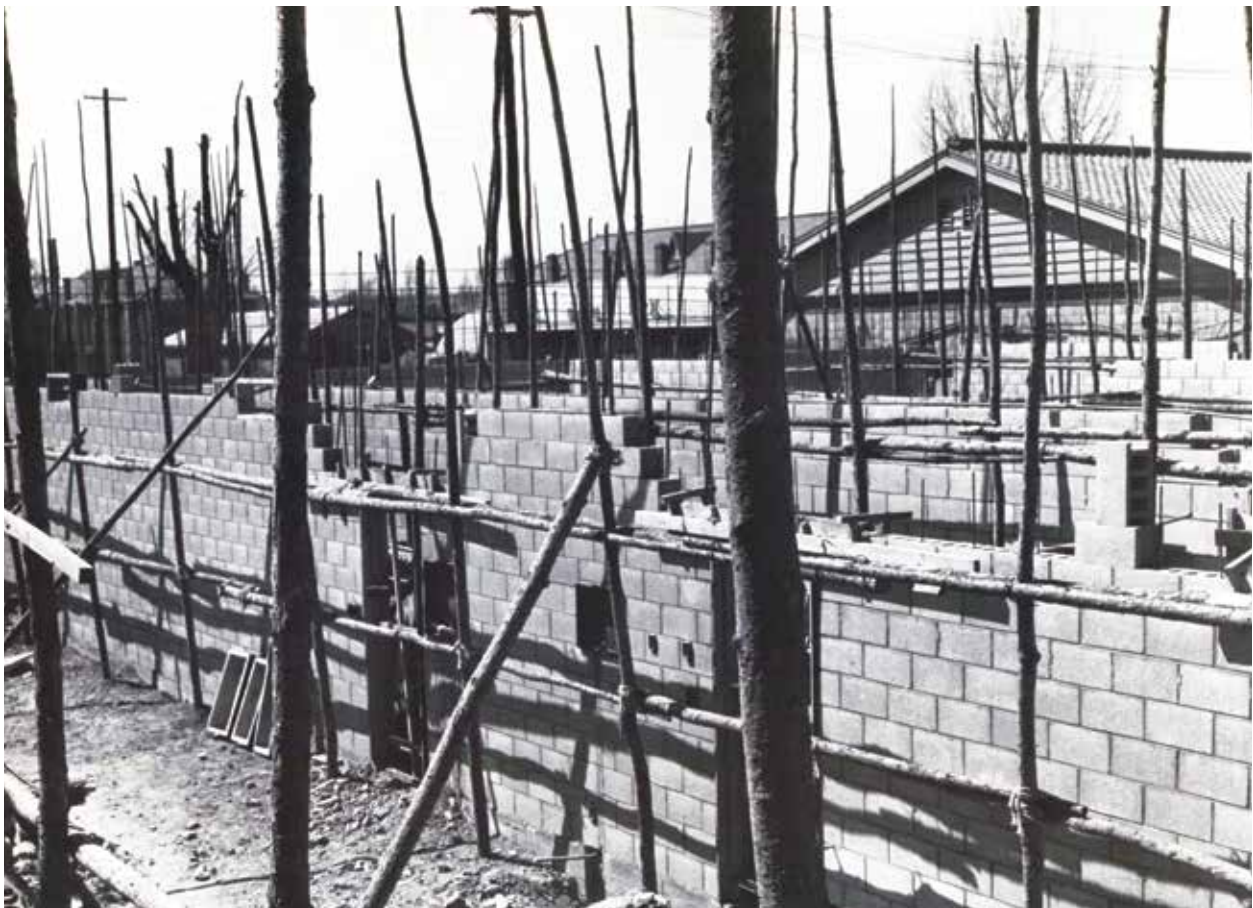
Concrete-block walls and scaffolding used to build the ACAN (Army Command Administrative Network) Communications Center, Seoul Area Command, April 1960.
