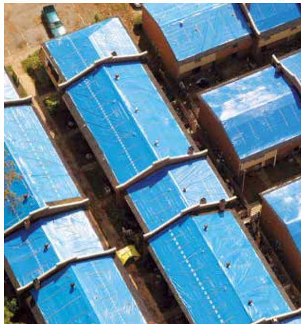
Operation Blue Roof helped to prevent further damage to structures as a result of Hurricane Katrina. Credit: John Fleck / FEMA
