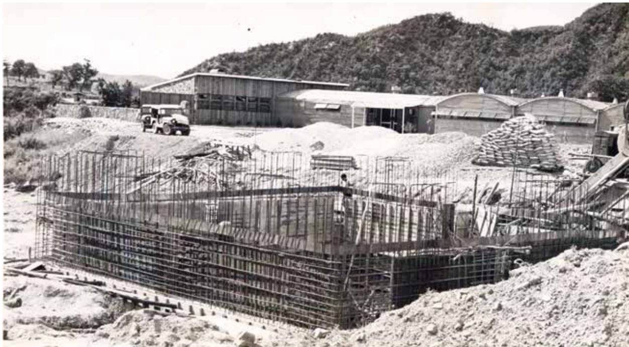
An early FED project: Construction of a water supply system at Camp Saint Barbara, in the forward area, August 1957.
