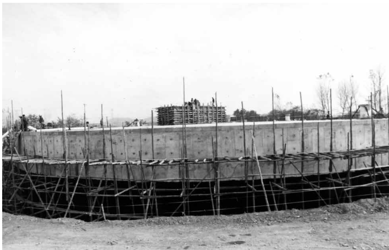
Construction of a 100,000-barrel jet fuel storage tank at Kwangju Air Base, 1983.
