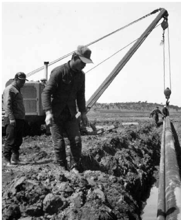
Pipeline casing being lowered into a trench, April 1969. Credit: NARA RG 111, CC-56300
