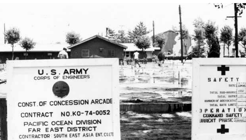
Workers using a pile driving machine during construction of troop housing at Camp Humphreys in the 1970s.
