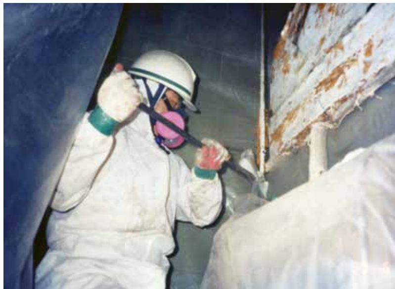
An FED contractor pries asbestos laden material from a wall in the 1990s.
