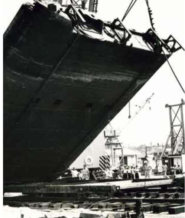
Removal of one of the 100-ton miter gates at the Incheon Tidal Basin, October 1959. Credit: Photo by Sergeant Ray Boswell, FED, PAO-FED Historical Files
