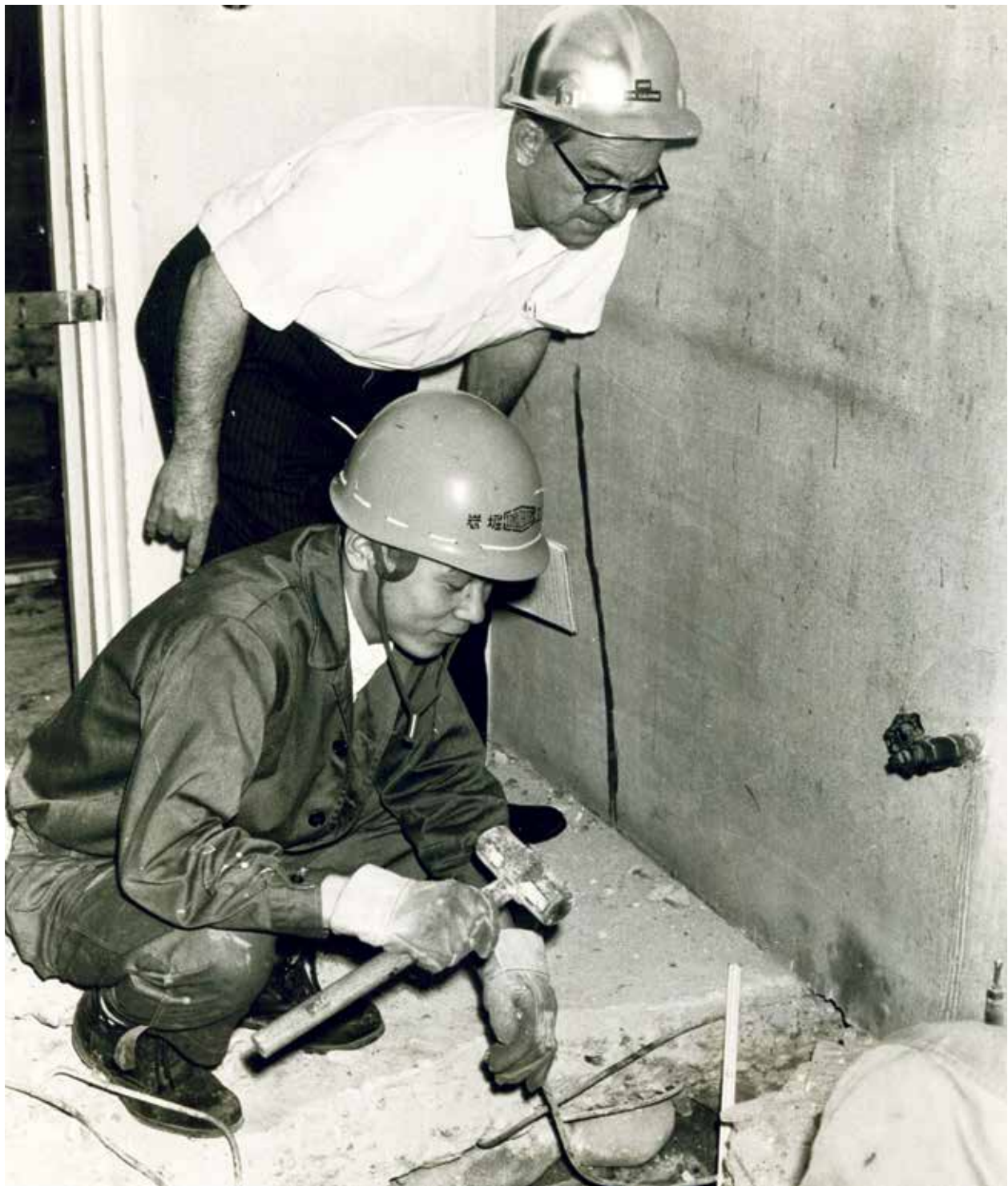
FED's Jim Calhoun checks on the progress of an operating room being built at the 106th General Hospital at Kishine Barracks, near Yokohama, May 1966. Credit: Photo by SP5 Mike Fournell, U.S. Army, FED-PAO Historical Files.
