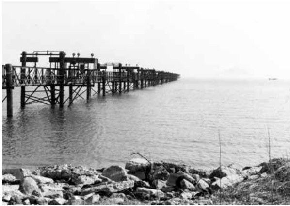
Light pier to help guide airplanes at the approach to Kunsan Air Base, 1972-1974.
