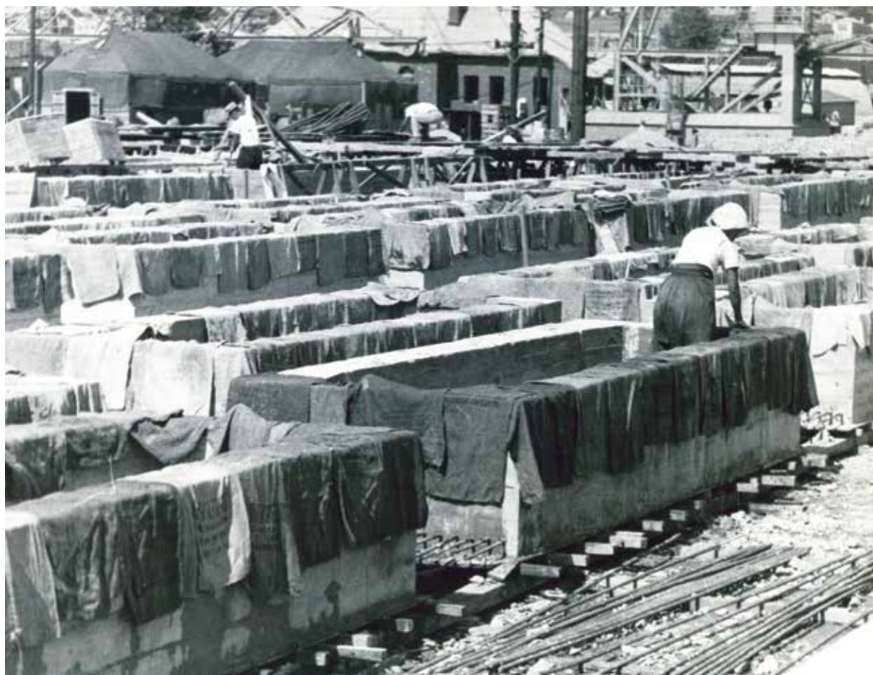
Korean workers curing the precast concrete floor beams used to repair the south wharf of the Incheon Tidal Basin, November 1959. Credit: Photo by Sergeant Ray Boswell, FED, PAO-FED Historical Files
