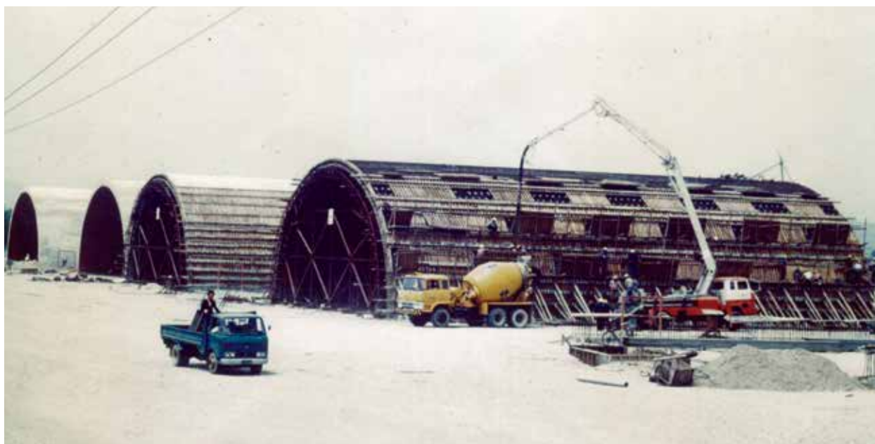
Quick-turn aircraft facilities at the Suwon Combined Defense Project, 1984.
