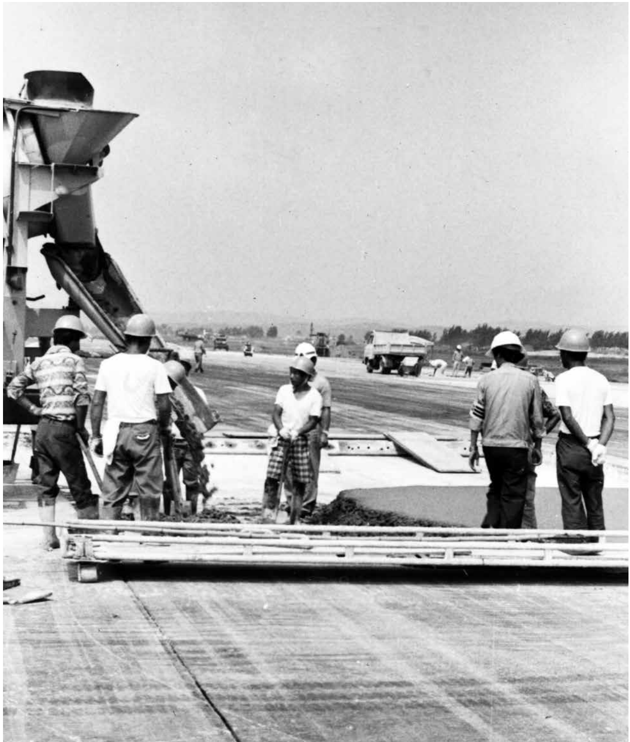
Workers for FED contractor Pum Yang pour new asphalt pavement for the runway at Osan Air Base, during the 100-day shutdown in summer 1983.
