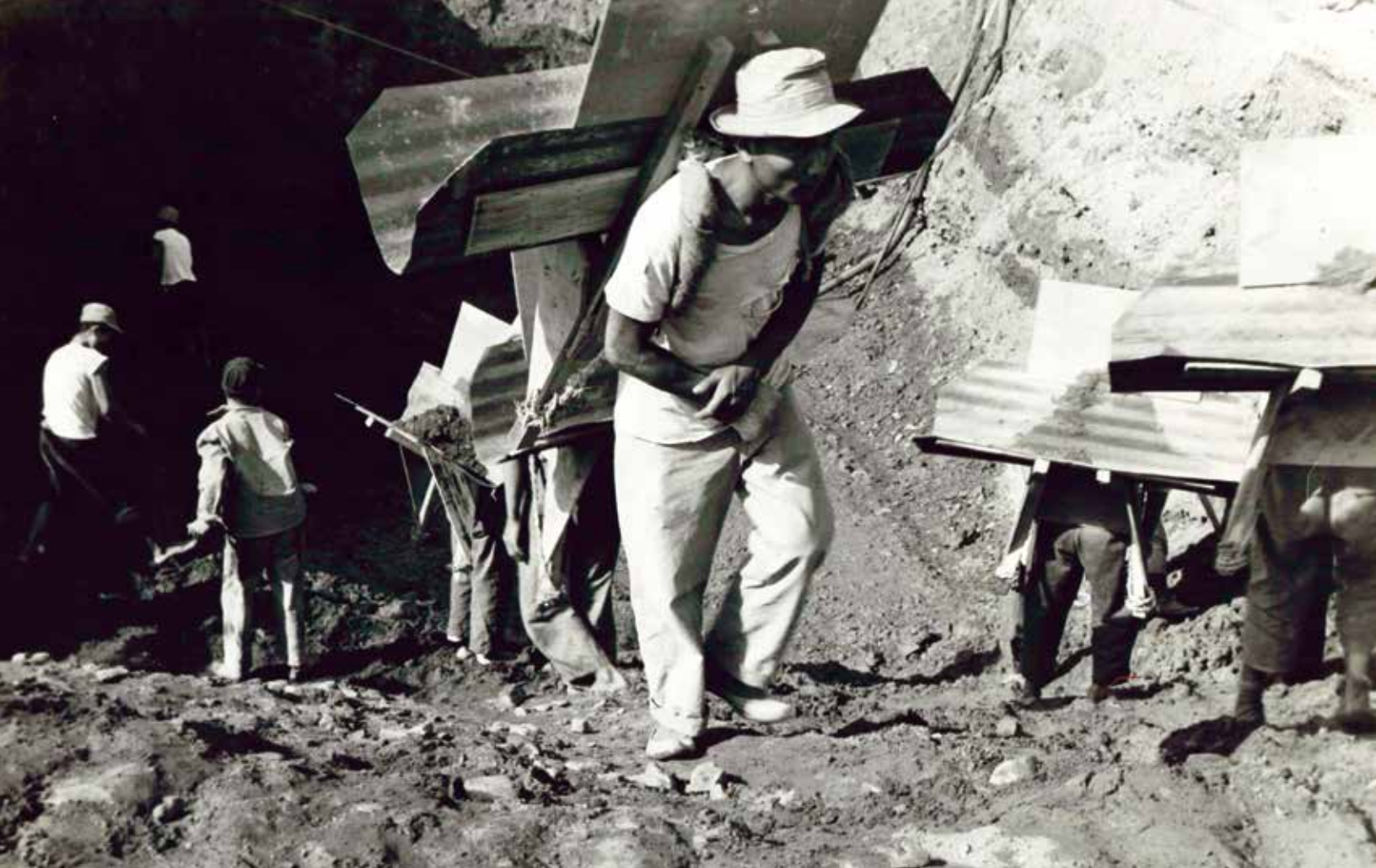
Korean laborers hauling dirt using modified A-frames, at Seoul Area Command Special Services Building, October 1960.
