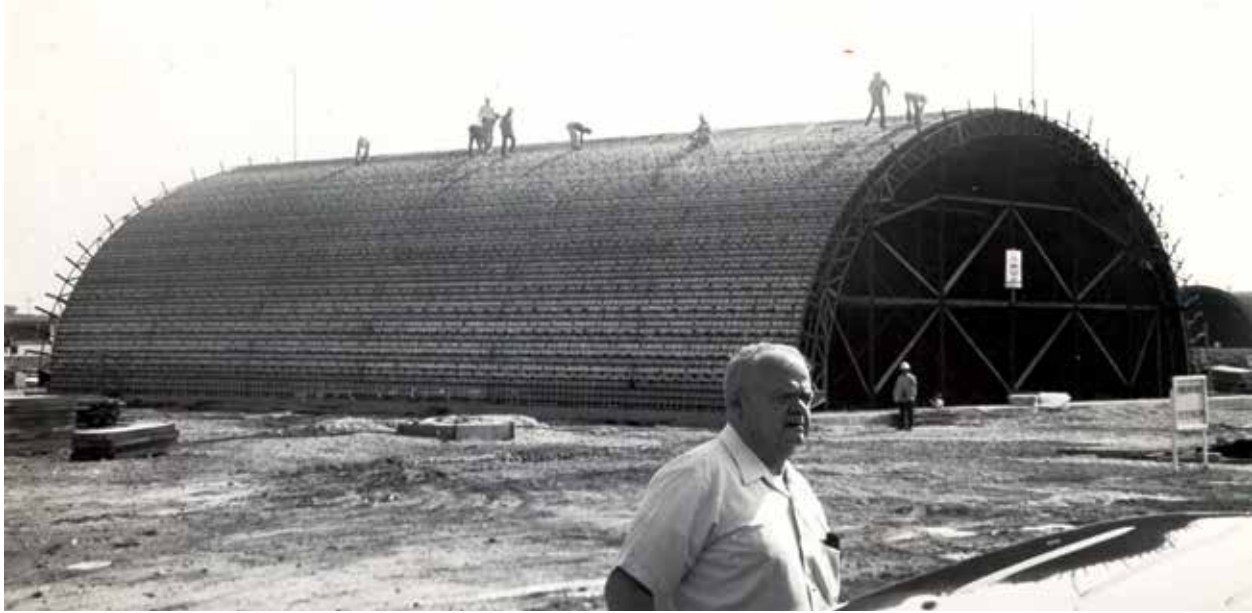
Quick-turn aircraft shelter under construction at Osan Air Base, June 1983, with FED's Howard Elliott in the foreground.
