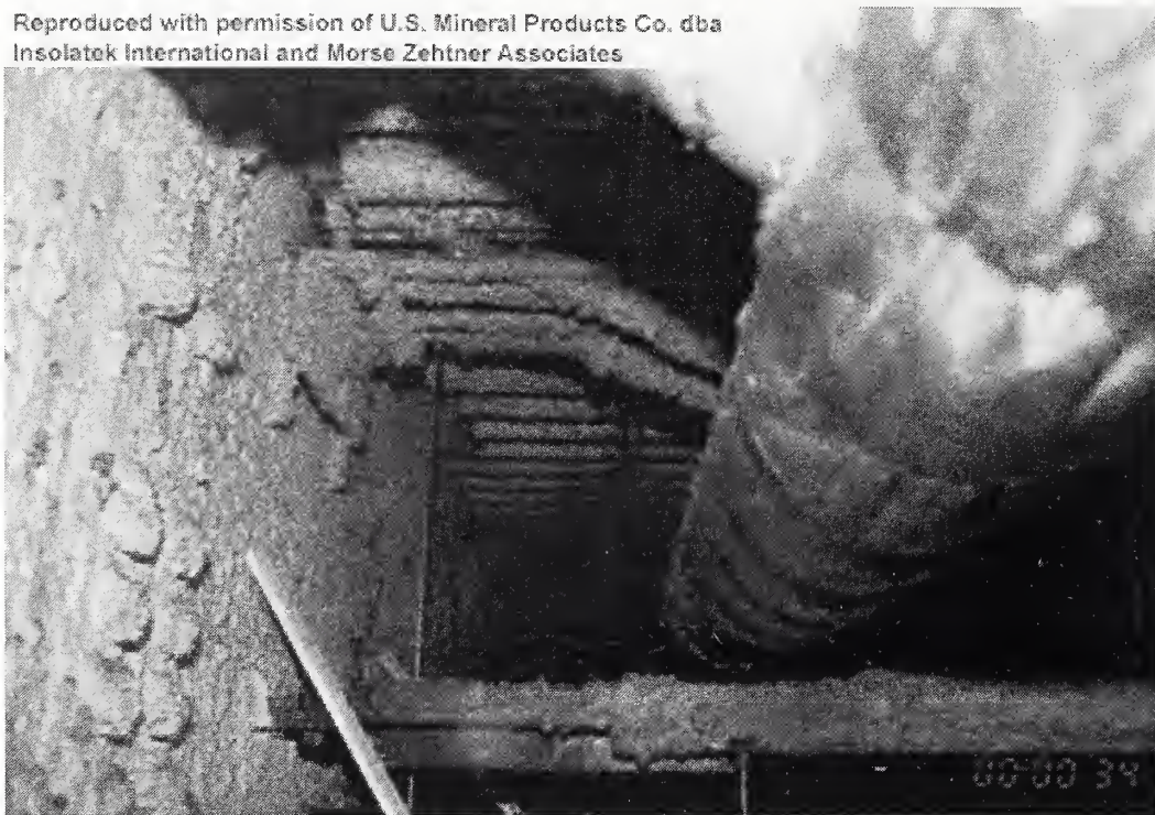
Figure 3–7. Connection of main truss to spandrel beam showing relatively thin SFRM on truss seat and no SFRM on damper.
