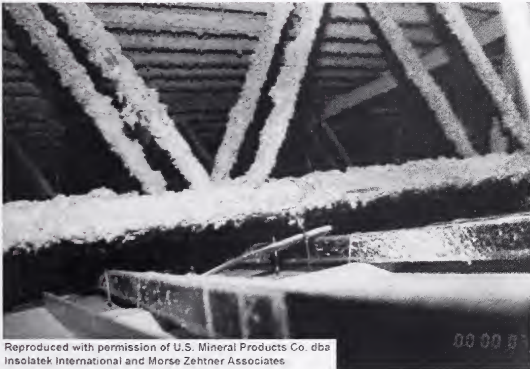
Figure 3-10. Example of damage to SFRM during installation of utilities.
