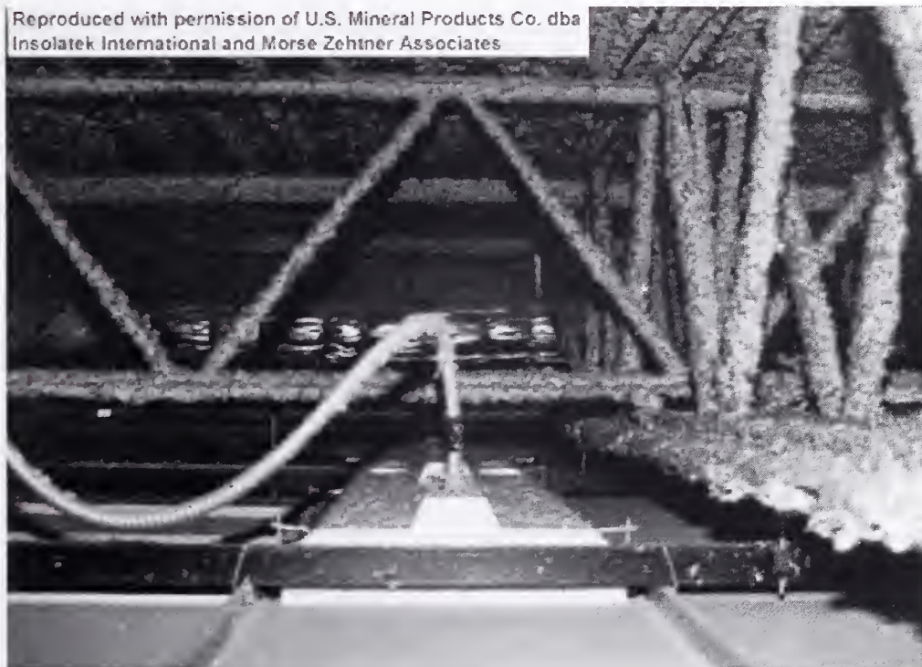
Figure 3–6. Intersection of main truss and bridging truss showing thinner SFRM on members of bridging truss.
