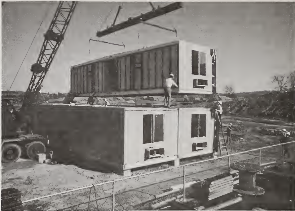
Figure 2: Air Force housing module. Sidewalls have sheathing only on inner face of steel studs.
