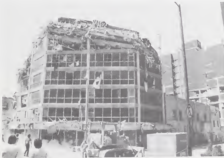
(b) Upper story failure in clothing store.
