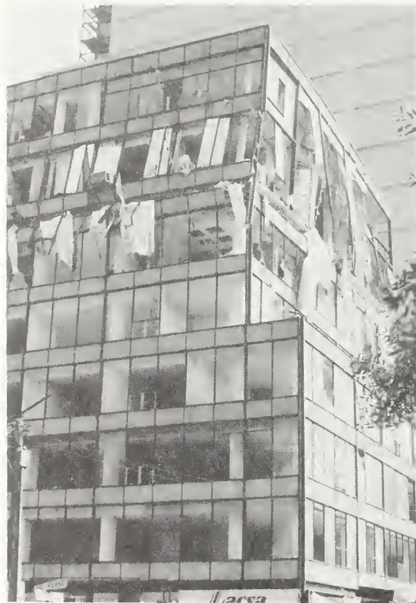
Figure 5.68. LASCA Building on Paseo de la Reforma and Marne, showing large change in column stiffness in upper two floor penthouse.
