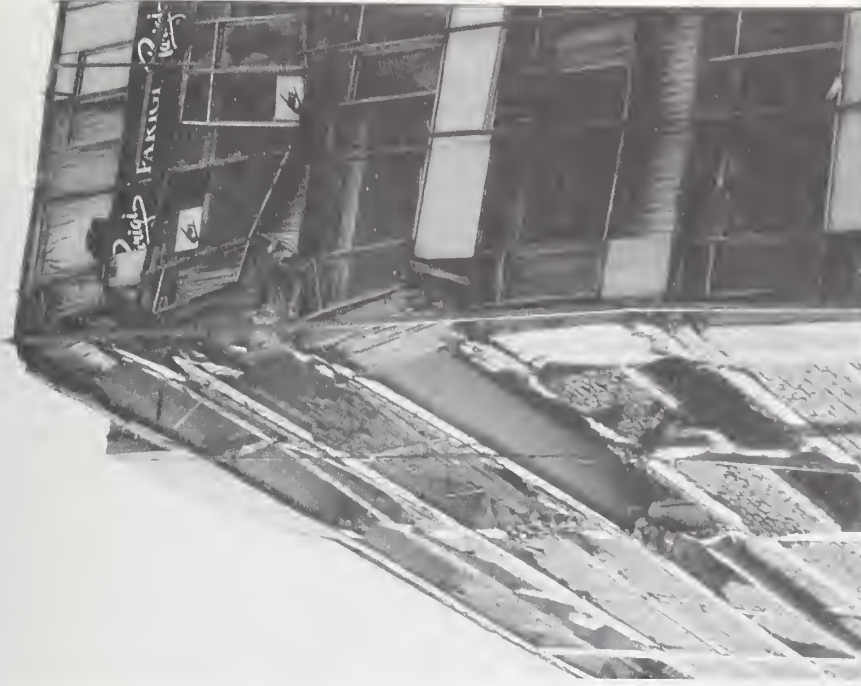
(b) Neighboring nine story building showing impact damage to columns.
