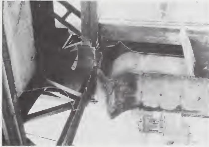
(a) Detail of the moment resisting connection of truss beam to column. (courtesy Dr. R. Hanson)
