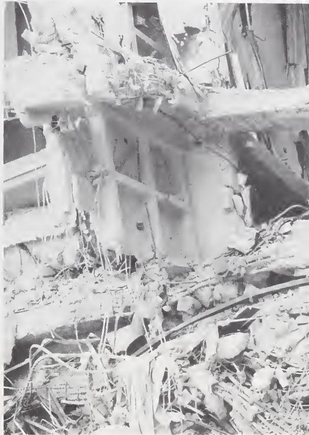
Figure 5.39. Collapsed 10 story apartment building in the corner of Dinamarca and Chapultepec. This waffle slab structure failure is attributed to base column failure and possible pounding with the neighboring structure.
