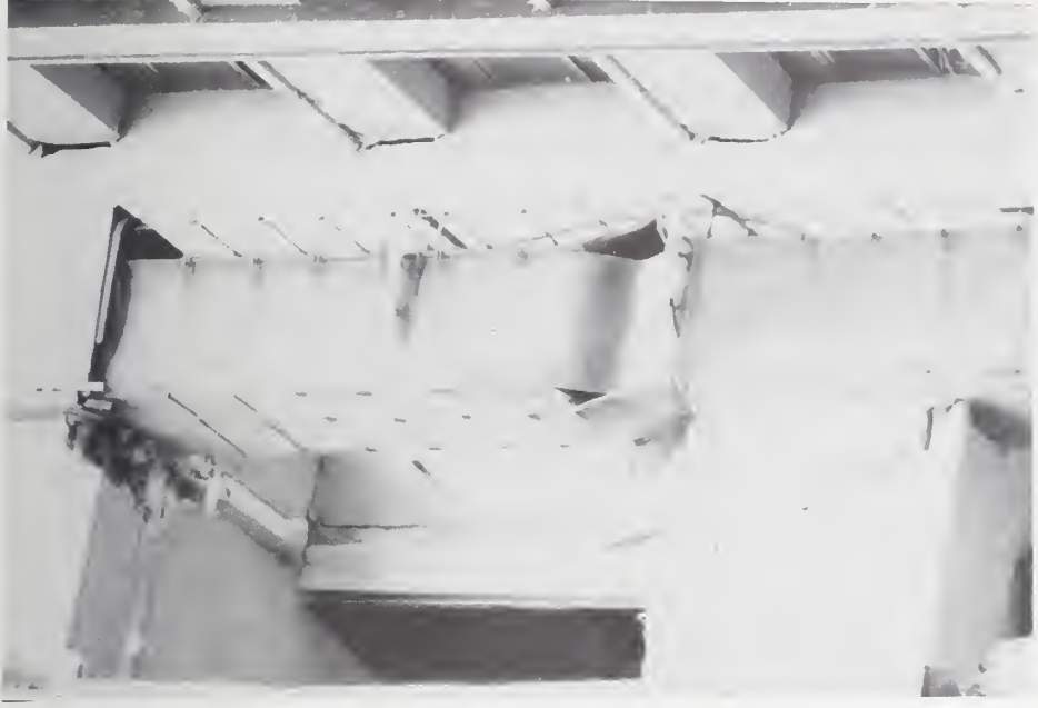
(b) Buckled column on south side of center 23-story tower. (courtesy E. Martinez Romero)
