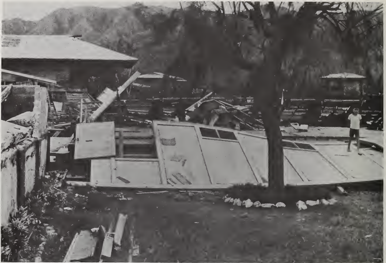
Researchers perform post-disaster surveys of building failures in foreign countries to improve building practices.
