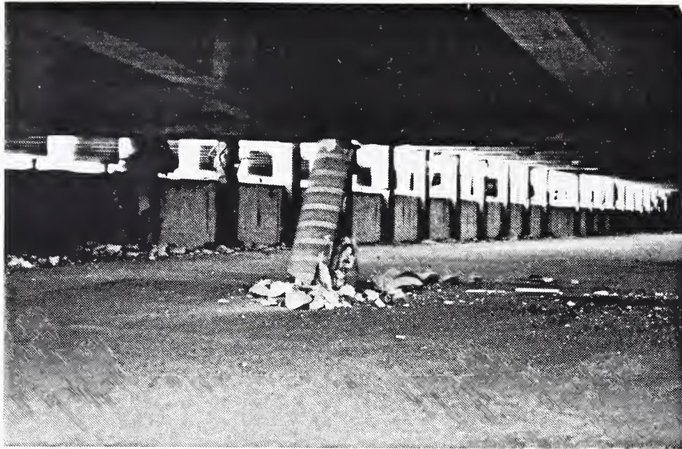
Photo 31 Non-ductile failure of a concrete column in the garage structure.
