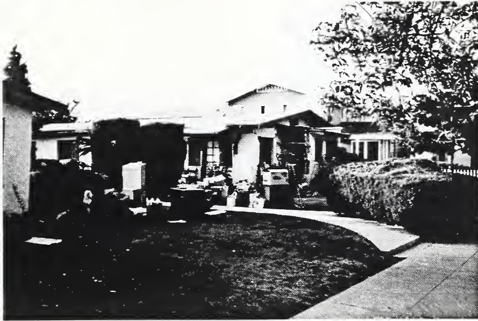
Photo 9 This house on Greenleaf Avenue lost part of the entrance and sustained severe cracks in the walls of unreinforced hollow clay tile.
