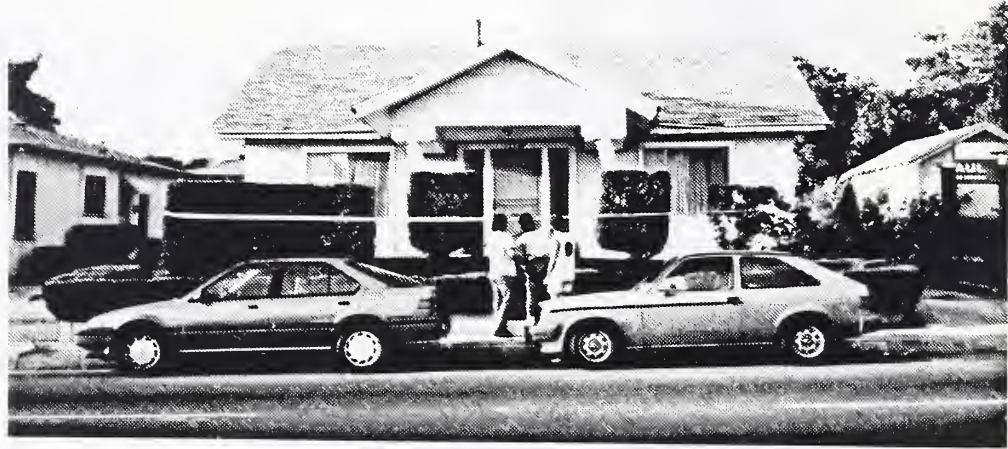
Photo 11 A wood-frame house on Beverly Blvd., Whittier, was damaged severely when it slid off its foundation wall.
