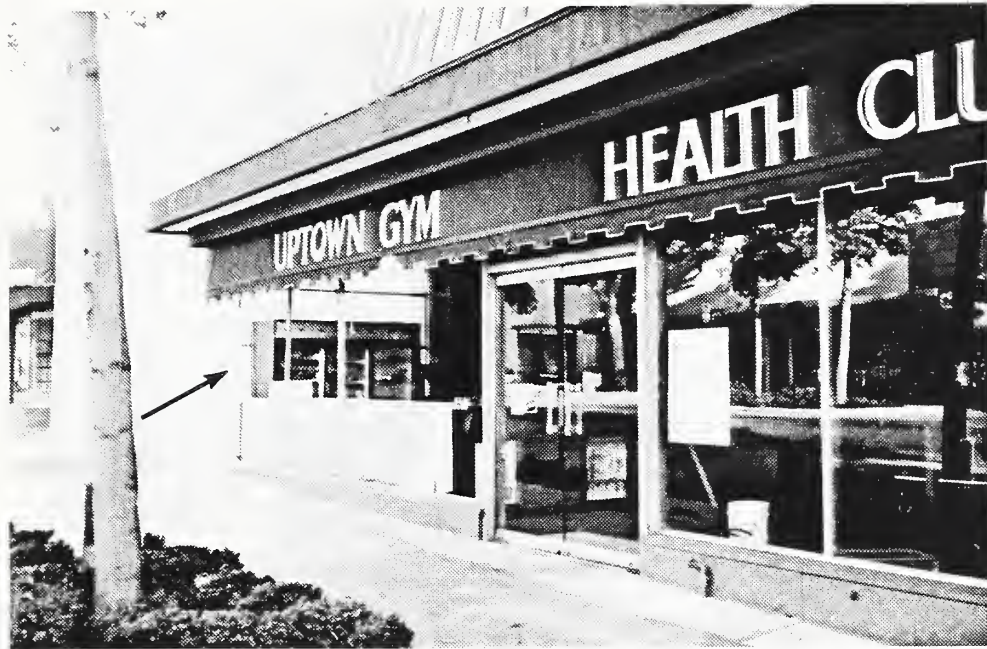
Photo 33 Distortion of the building caused damage to windows at the corner of the building in the Uptown Whittier shopping section.
