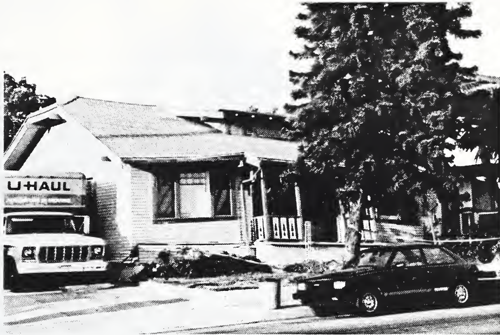
Photo 13 A wood-frame house adjacent to the house in Photo 11 on Beverly Blvd., Whittier, also sustained severe damage when the earthquake dislodged the house from its foundation wall.
