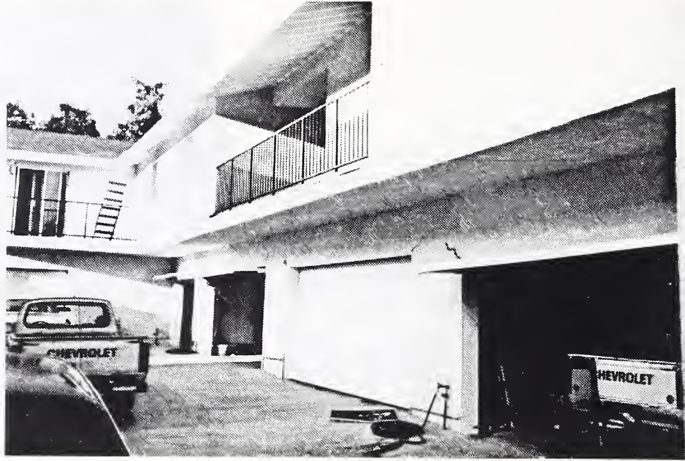
Photo 15 Damaged two-story wood frame apartment building in Whittier. Large garage door openings reduced the stiffness of the wall in the plane of the garage doors and reduced the resistance to lateral loads.
