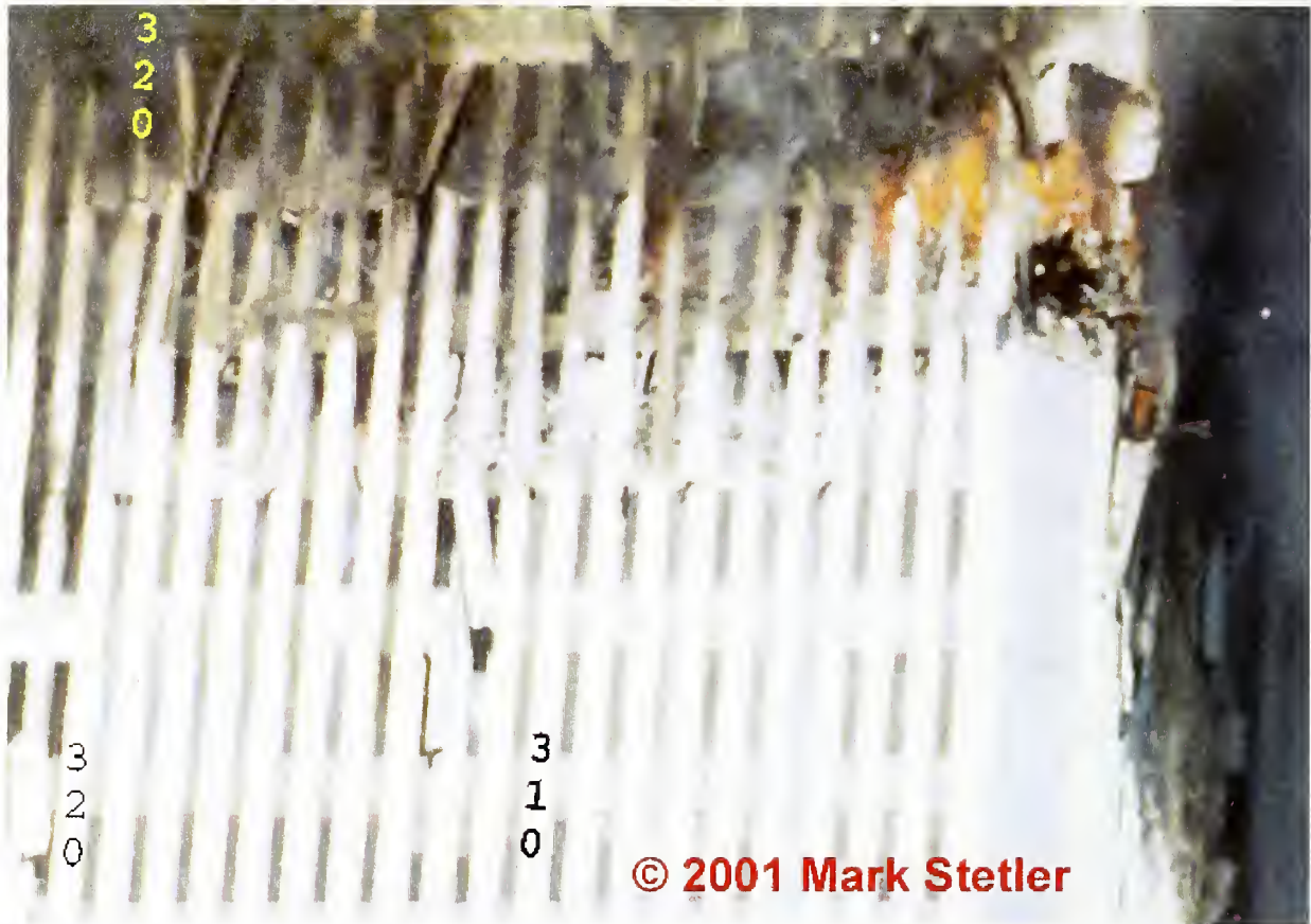
Figure H-7. This photograph is cropped from the image shown in Figure H-6. It was taken on September 11 and shows the east face of WTC 2 at the northeast corner from floor 77 to floor 82. Note the large piles of debris evident on floor 80 and floor 81.
