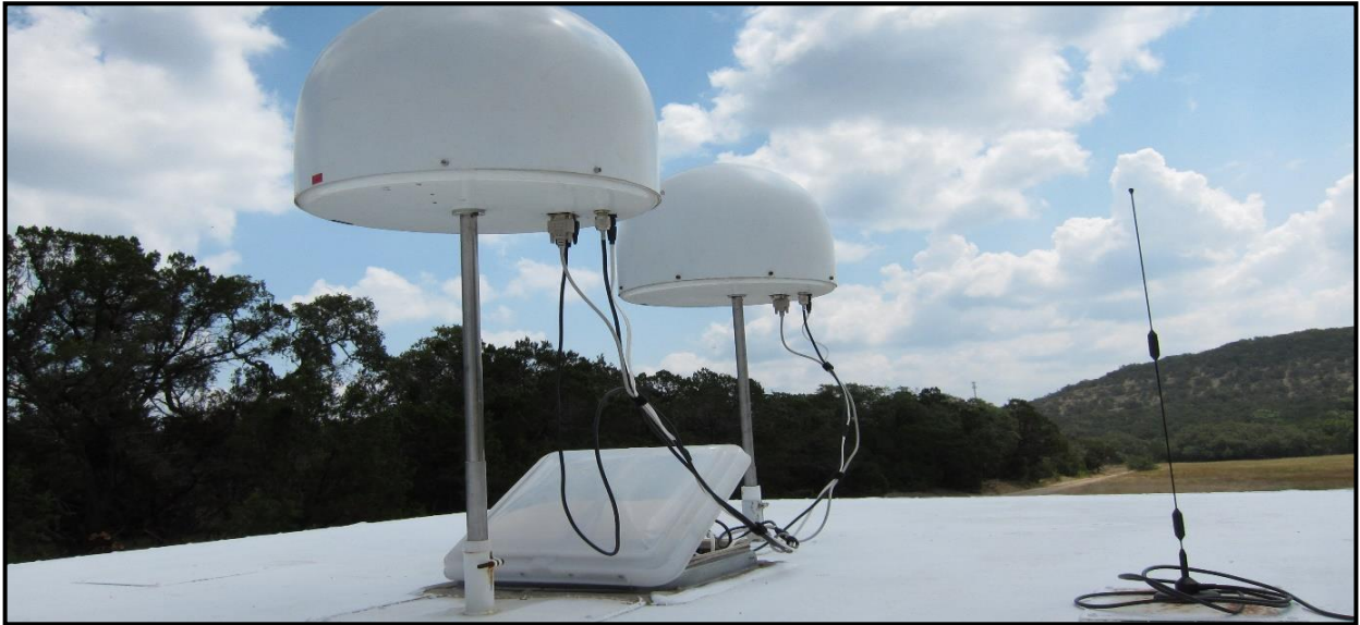
Figure 16: The radome and telemetry antennas in place on the trailer roof.
