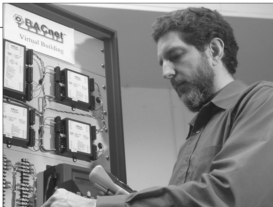
Steven Bushby, leader, Mechanical Systems and Control Group, checks wiring connections for controllers in the BACnet™ Virtual Building.
