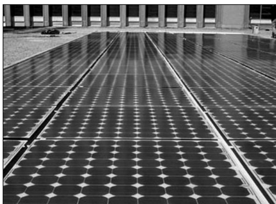
Photovoltaic Array installed on the NIST Administration Building that provided NIST's first on-site renewable energy on 14 September 2001.
