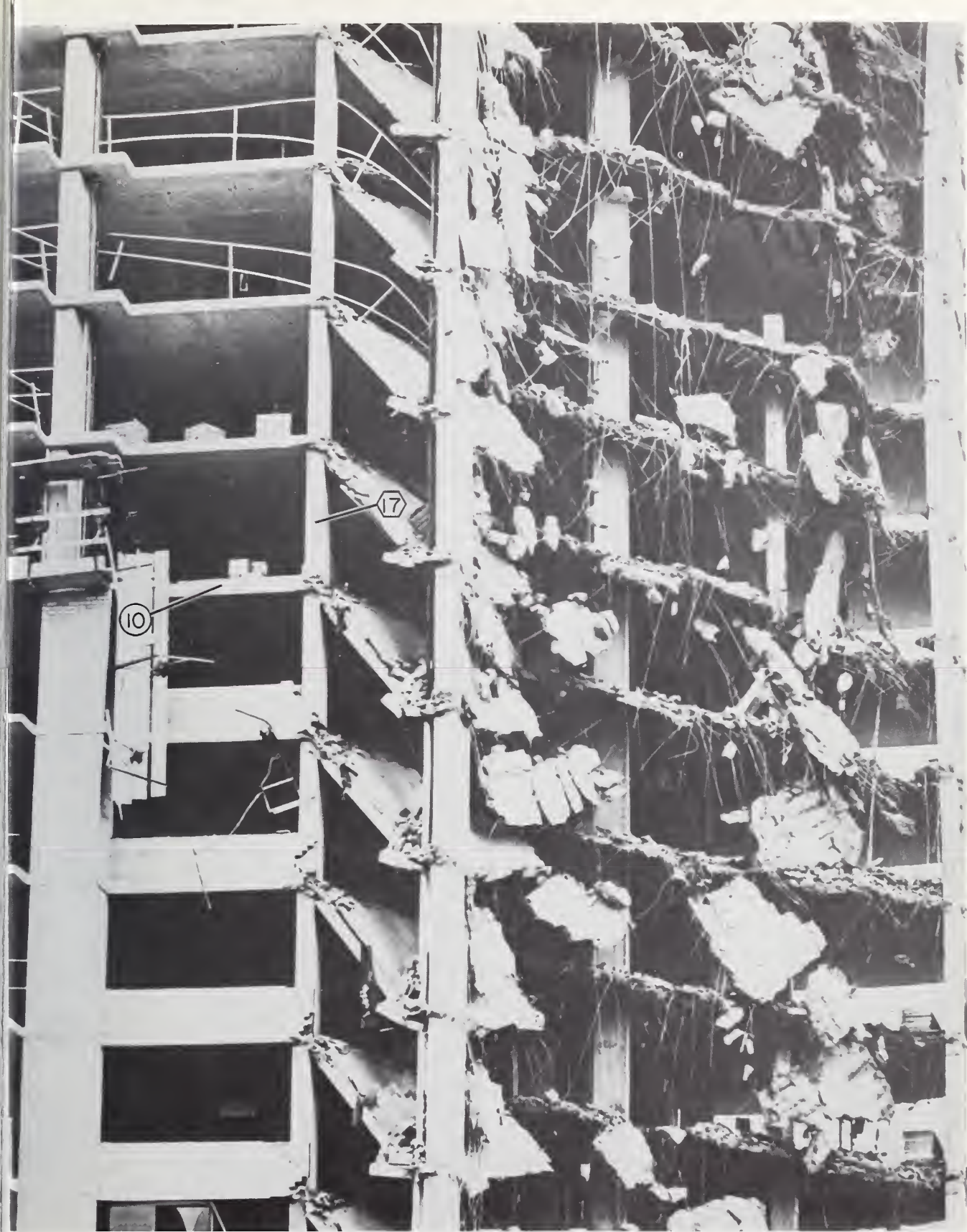
Figure 2.8 Closeup view near the midheight of the east end of the failure zone looking south.
