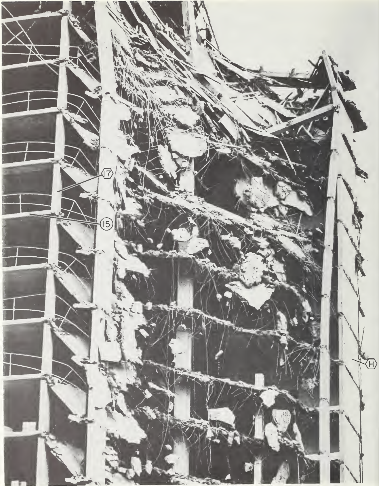
Figure 2.7 Closeup view near the top of the east end of the failure zone, looking south.
