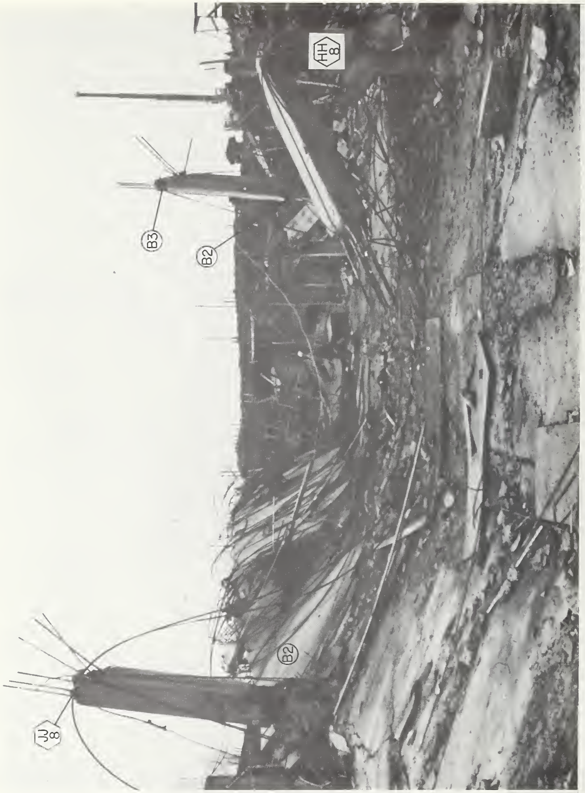
Figure 2.45 View looking west of slab B-2 between column lines HH and JJ.
