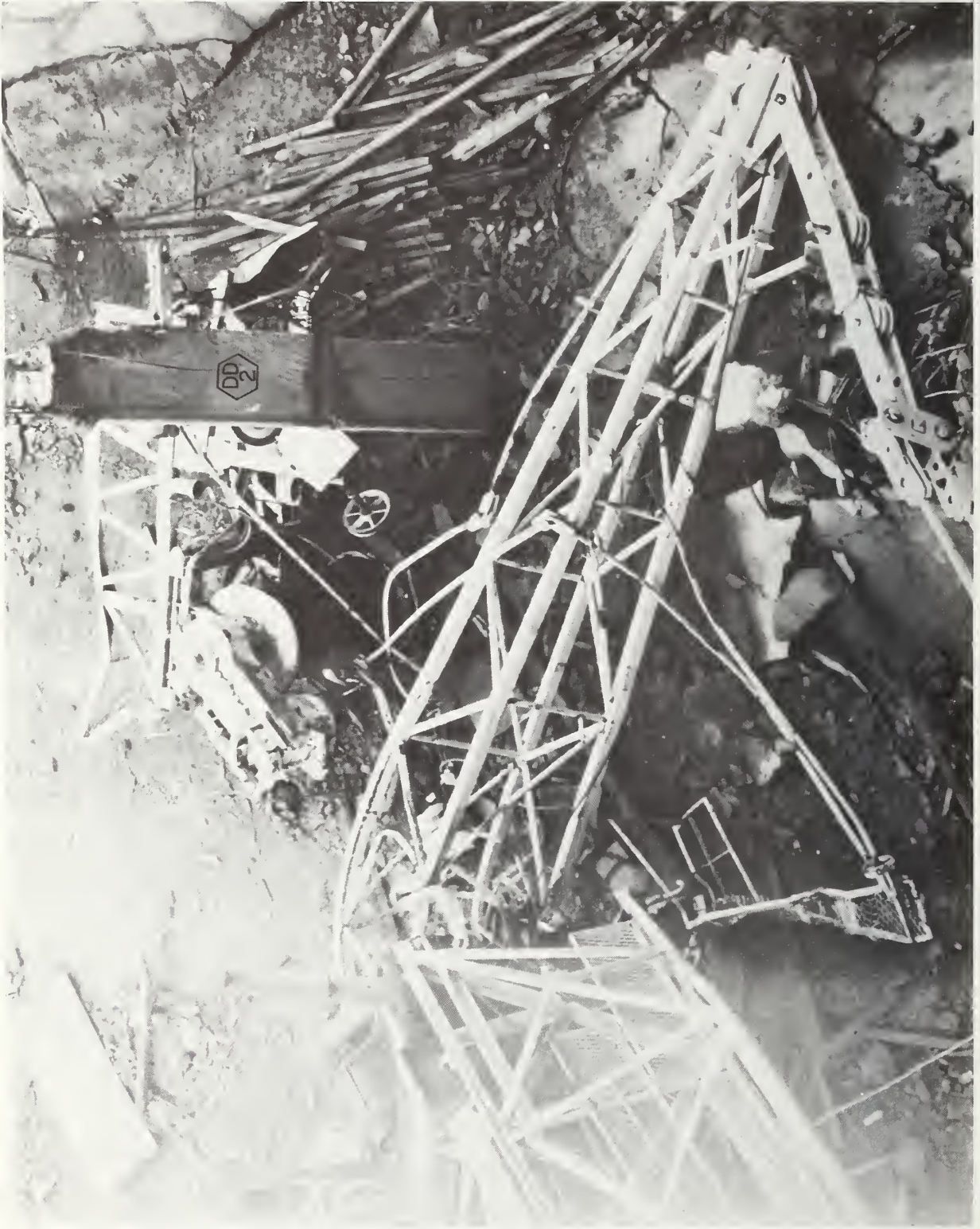
Figure 2.55 Position of fallen crane near column DD-2 looking south.
