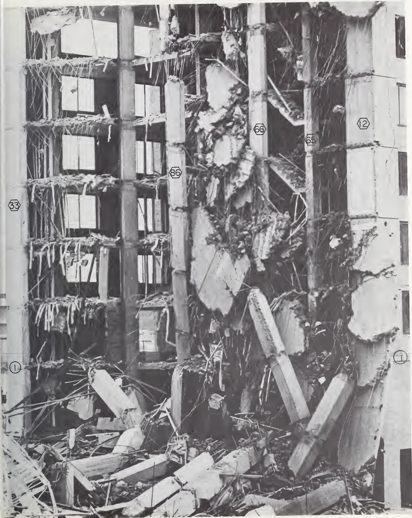
Figure 2.12 Closeup view at the bottom of the west end of the failure zone, looking southwest.
