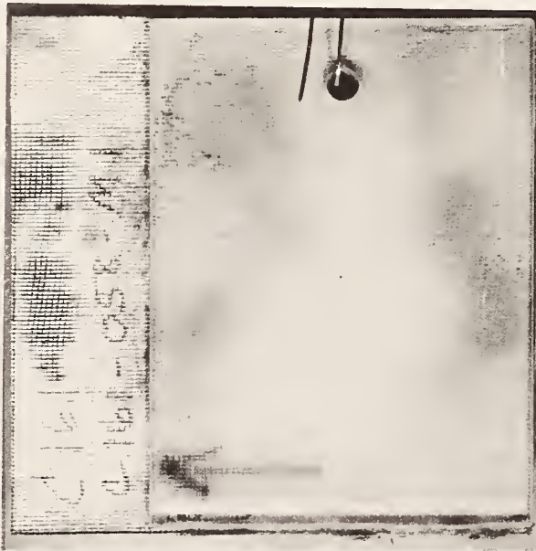
Figure 6. An example of fungal growth on the exposed backing material (left side) and in the adhesive between the wallcovering and the glass.
