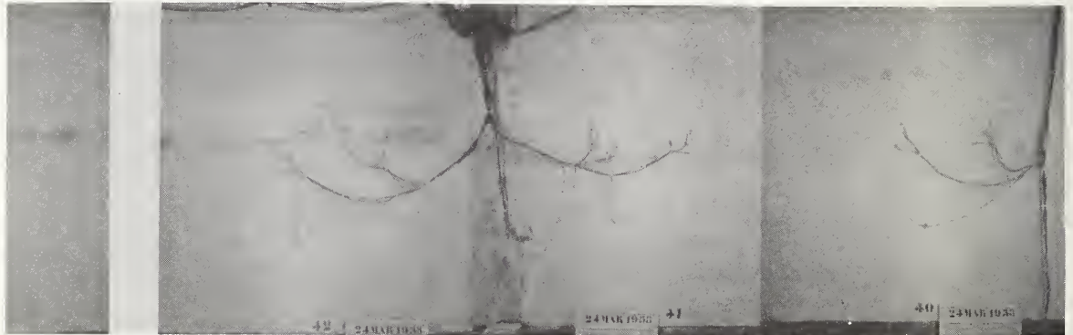
Interior view, condensation on the reactive paint
