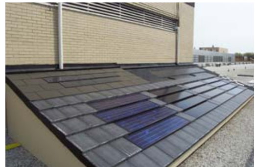
NIST's outdoor residential photovoltaic test facility is used to collect performance data for model improvement and validation. (Photo: NIST)
