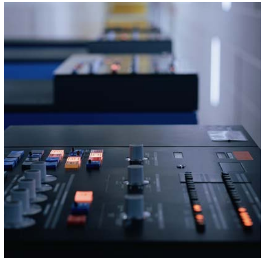
Commercial building systems control panel. (Photo: MS Online)
