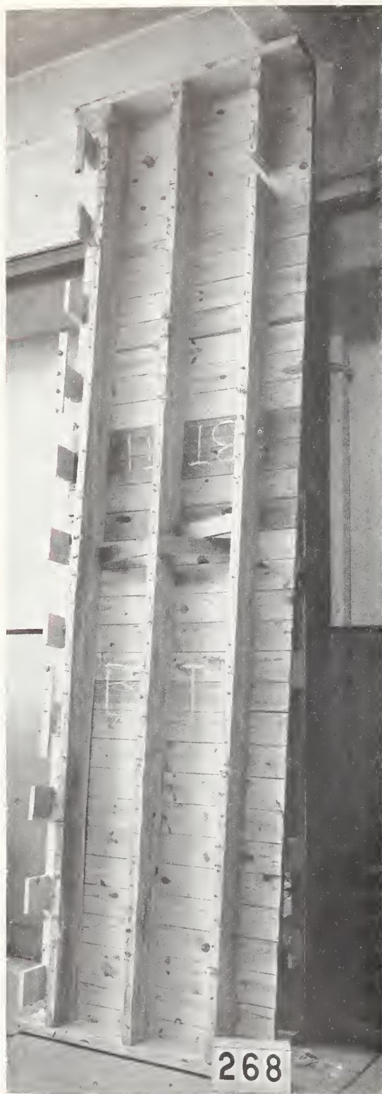
FIGURE 4.—Roof BT. Typical specimen.
